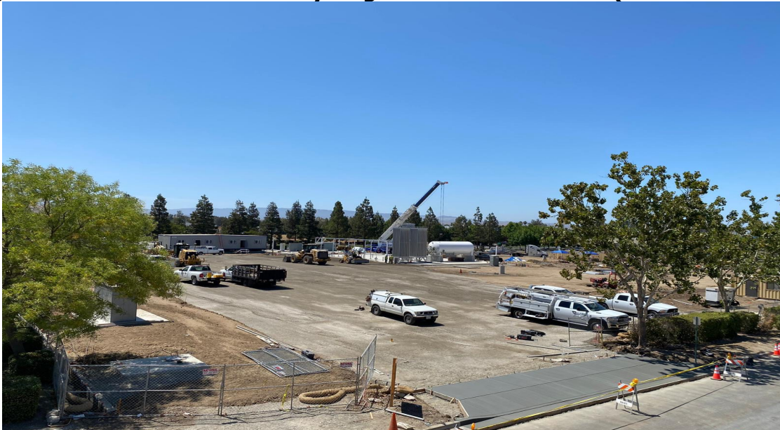
Figure 12: FirstElement Fuel Hydrogen Hub in Livermore (Alameda County)
