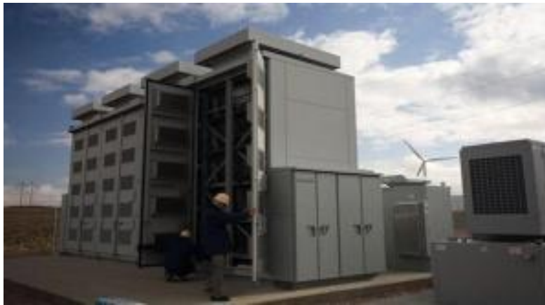
Figure 3 Lead-Acid Battery Storage
