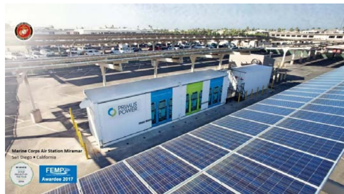
Figure 5: Primus Power Flow Battery Installed at Marine Corps Air Station Miramar
