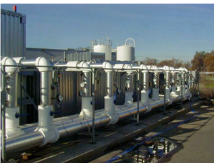
600 gallons of ice storage used to shift peak electrical loads to off-peak period.
