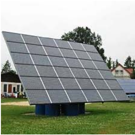
Solar generates electricity to run pump
