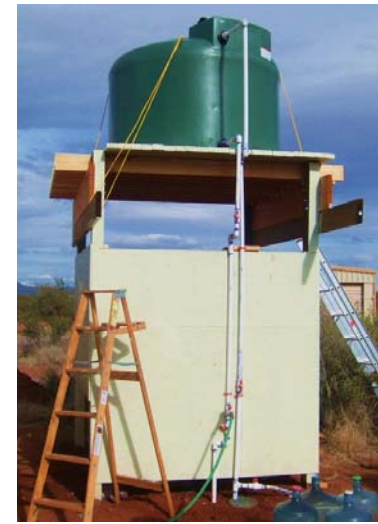
Pump stores water at elevation during day to water at night
