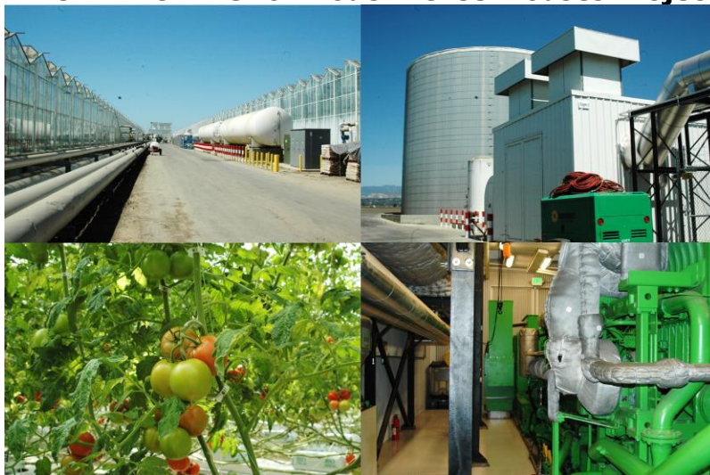
Figure 14: CHP with TES for Modern Greenhouses Project Photos
