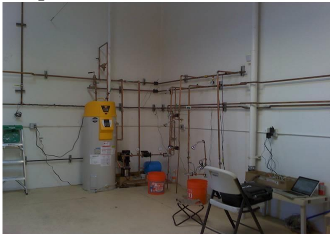
Figure 7: Testing Crossover and Unbalanced Recirculation Loops
