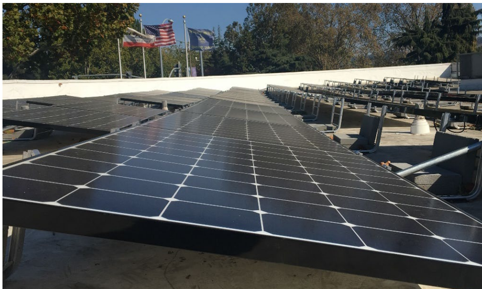
Figure 6: Solar PV Panels on Rooftop
