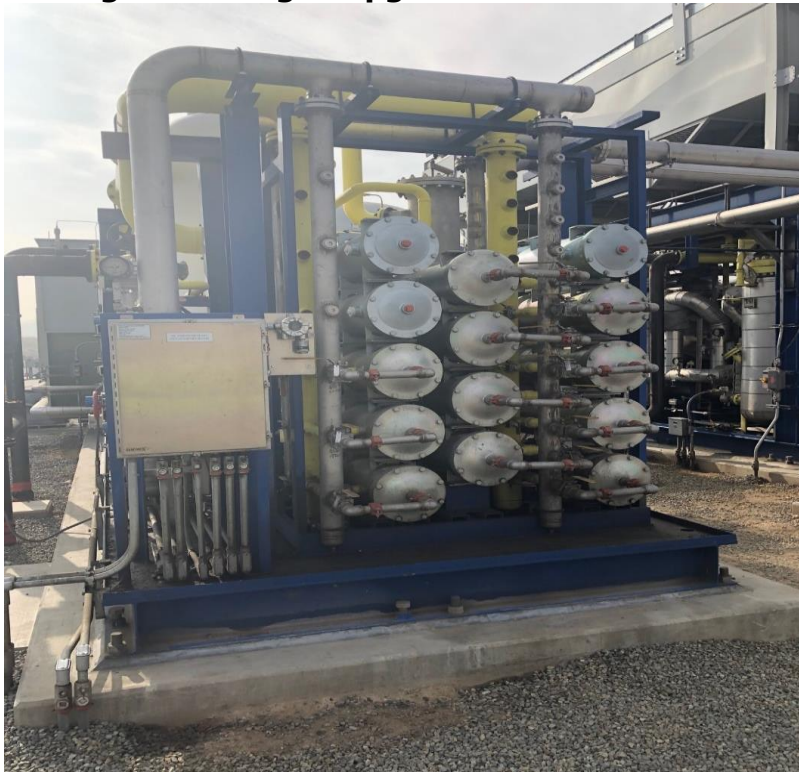
Figure 9: Biogas Upgrader Membranes #1
