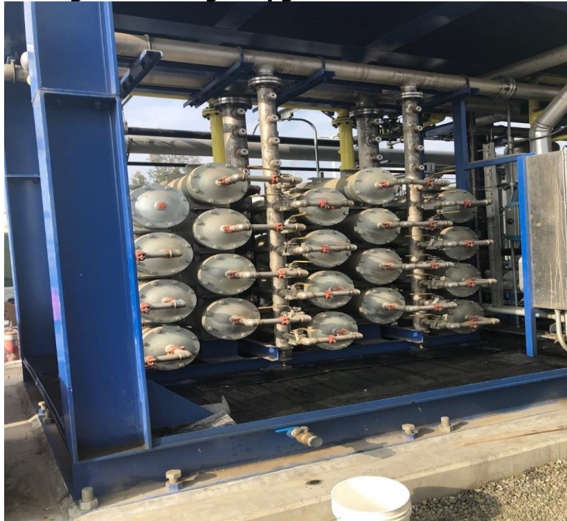
Figure 10: Biogas Upgrader Membranes #2
