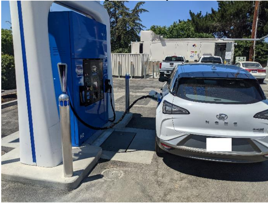
Figure 11: Customer Fueling at the Campbell East Hamilton Station
