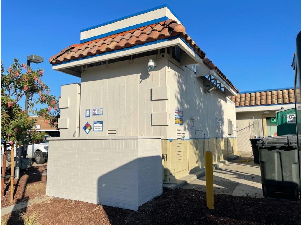
Figure 4: Linde Unit (Compressing and Dispensing Equipment)
