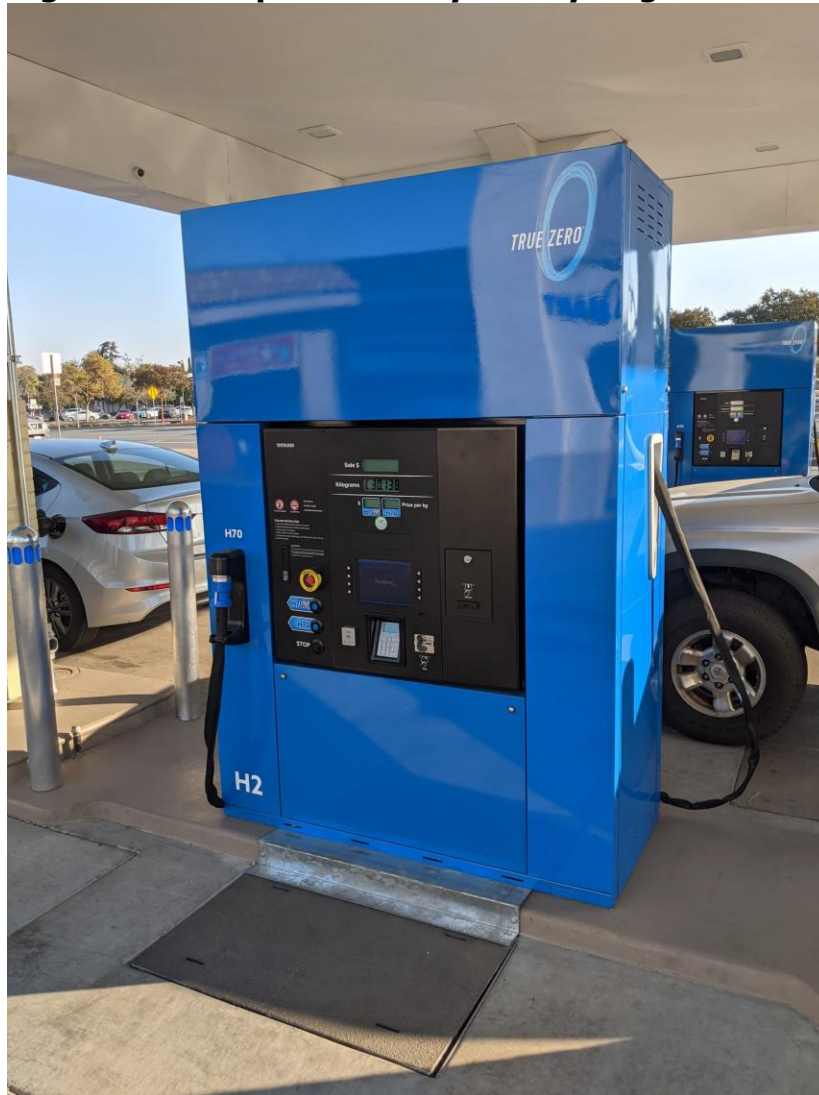
Figure 14: Completed Sunnyvale Hydrogen Station
