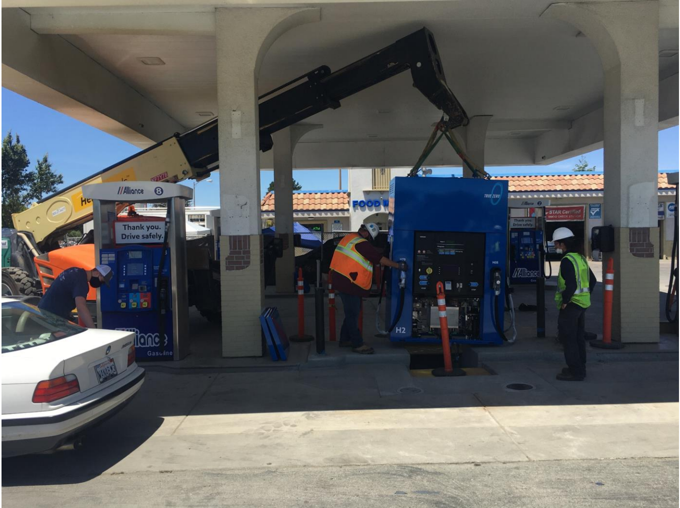
Figure 8: Tatsuno Dispenser installation at the Sunnyvale Station
