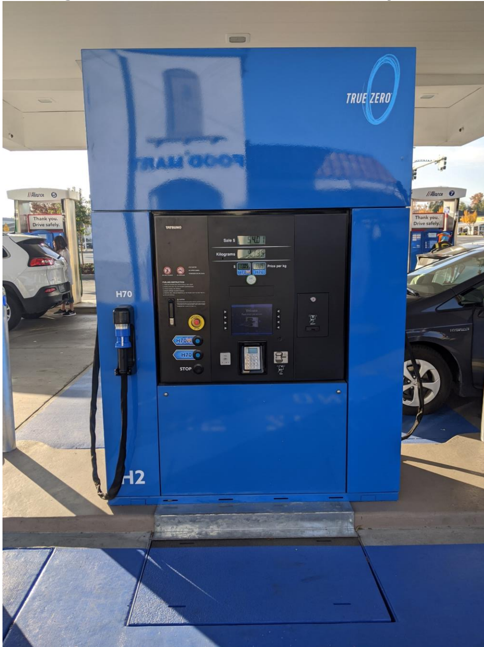
Figure 3: Installed Dual Sided Tatsuno Dispenser
