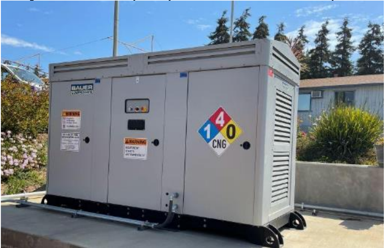
Figure 2: North Monterey County Unified School District's CNG Compressor
