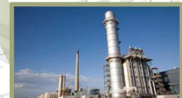
AUXILIARY GAS-FIRED BOILER
