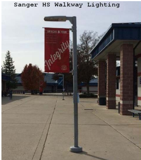
Figure 16: Sanger High School Walkway Lighting
