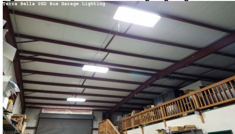
Figure 11: Terra Bella USD Bus Garage Lighting
