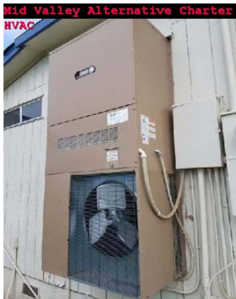
Figure 13: Mid Valley Alternative Charter HVAC
