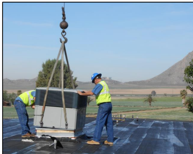
Photo Caption: HVAC being installed at Nuvview Elementary School in Nuevo, CA. Source: California Energy Commission
