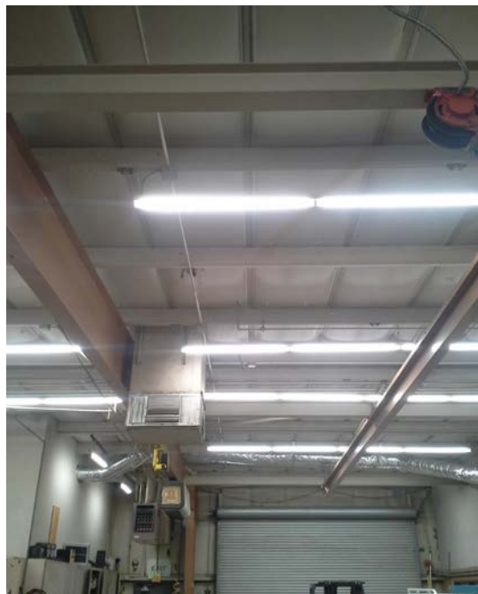
Photo Caption: LED Lighting installed at Kern Community College in Bakersfield, CA. Source: California Community College Chancellor's Office
