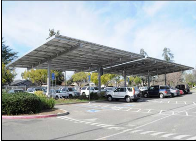
Photo Caption: Solar Panels Installed at Price Charter Middle School in San Jose, CA. Source: California Energy Commission
