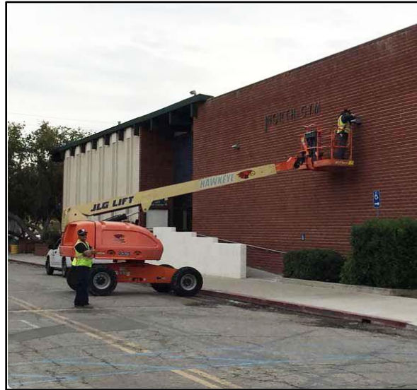
Photo Caption: New LED lighting being installed at El Camino Community College in Torrance, CA Source: California Community College Chancellor's Office
