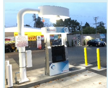
Photo Credit: Air Liquide
