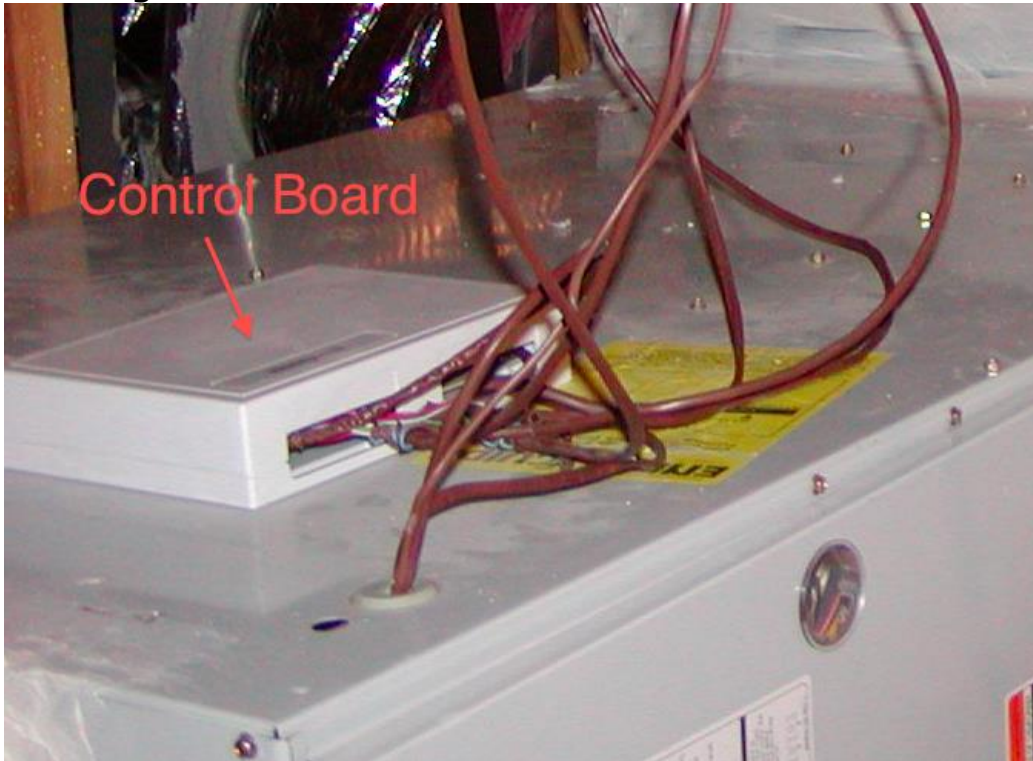
Figure 7: Photo of a cabinet-mounted control board.
