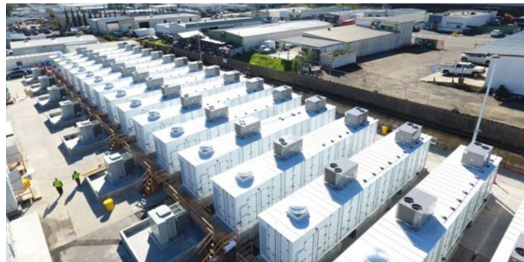
An energy storage project in SDG&E territory Credit: Cleantech San Diego
