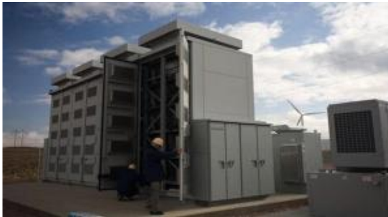
Figure 3 Lead-Acid Battery Storage
