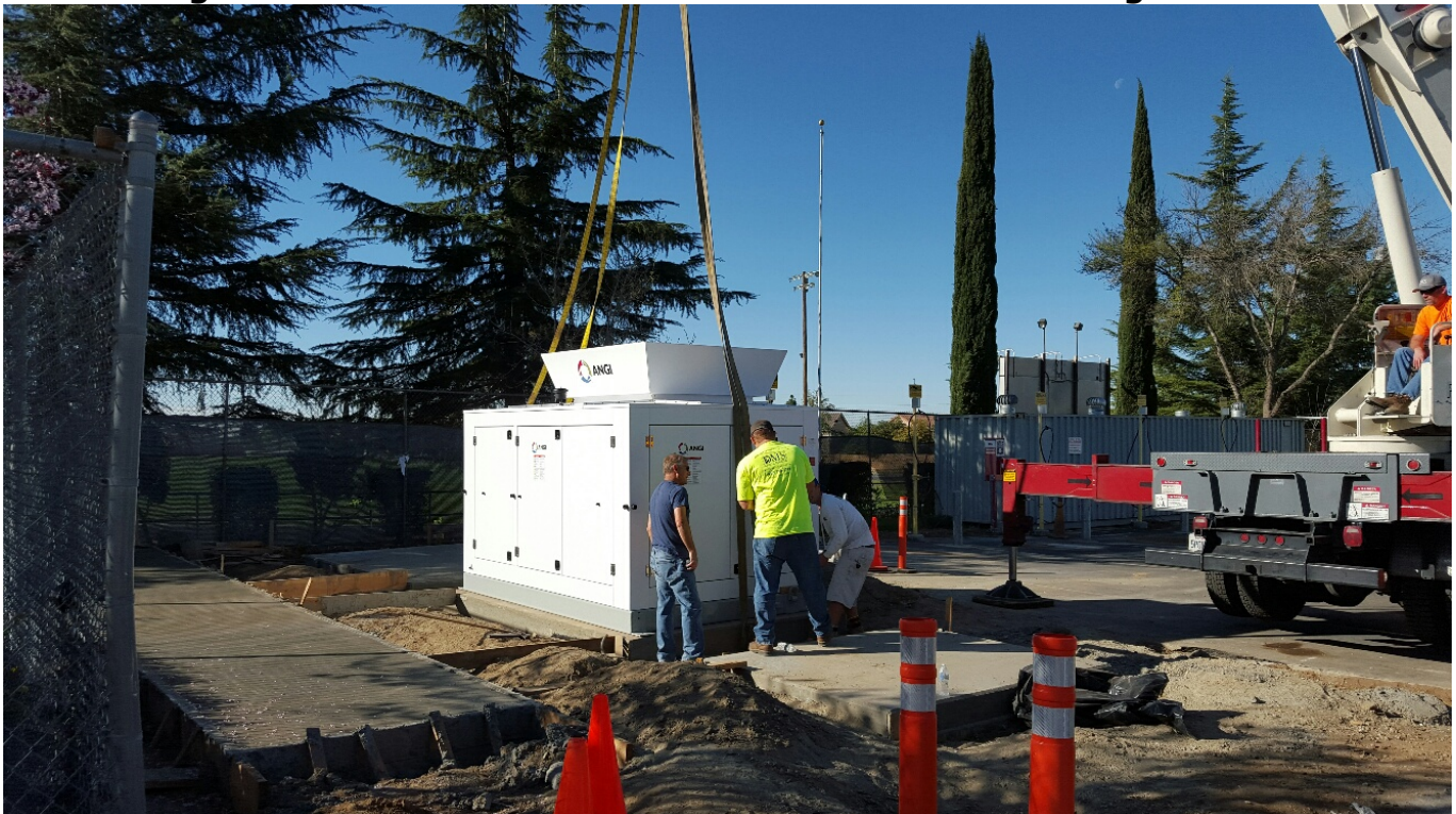
Figure 2: Beaumont Unified School District CNG Refueling Station
