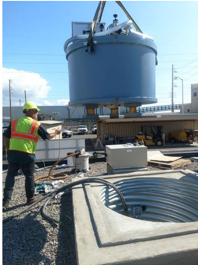
Figure 13: Demo for HECO at Campbell Industrial Park, Hawaii
