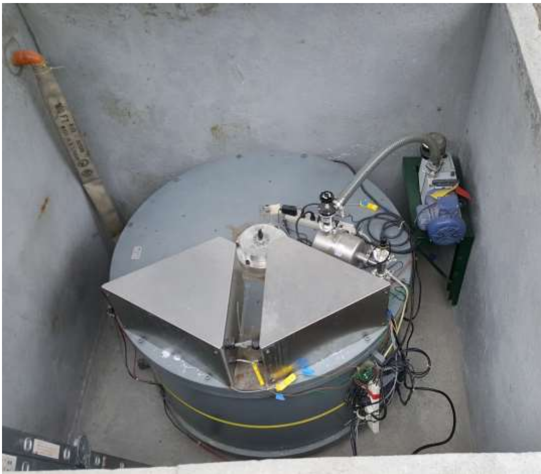
Figure 7: M25 Unit Installed in Original Containment Design
