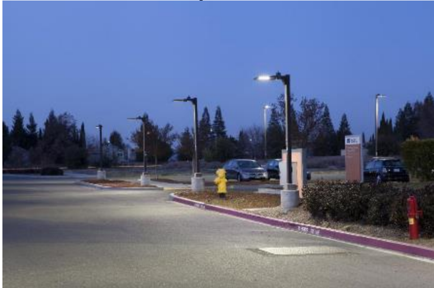
Figure 47: Light-Emitting Diode Parking Area Luminaries with Networked Control Systems
