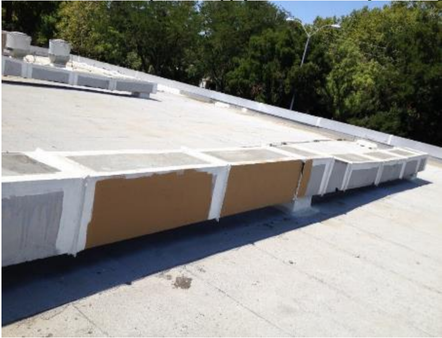
Figure 93: Pre-Retrofit of Exposed Supply Ductwork at Dry Cleaning Tenant
