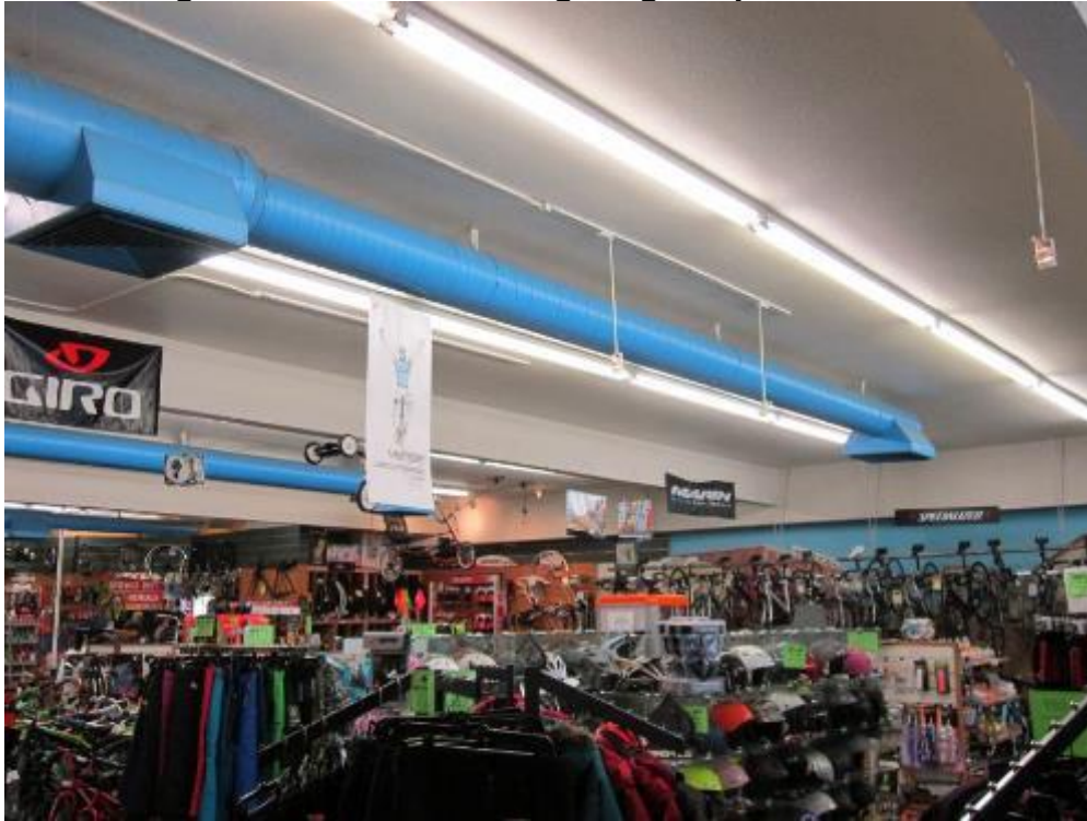
Figure 87: Pre-Retrofit Lighting at Sports Retailer
