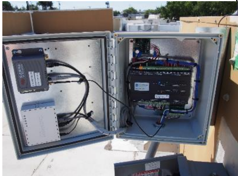
Figure 91: RTU Retrofit Control Box on Exterior of Rooftop Unit
