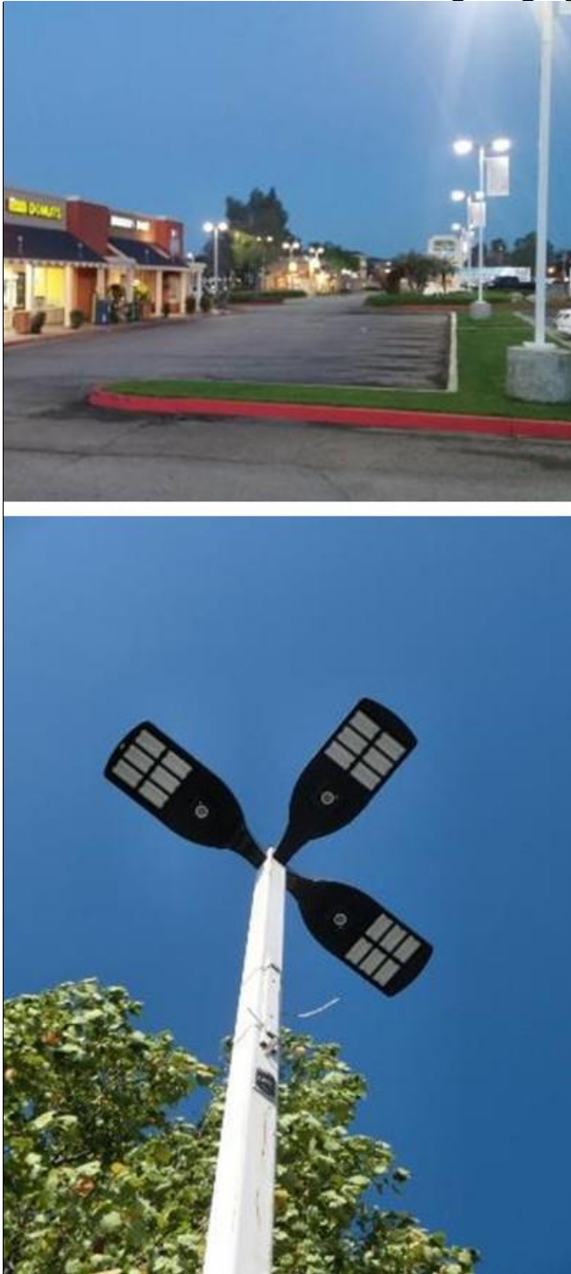
Figure 107: Post-Retrofit of Exterior Lighting System
