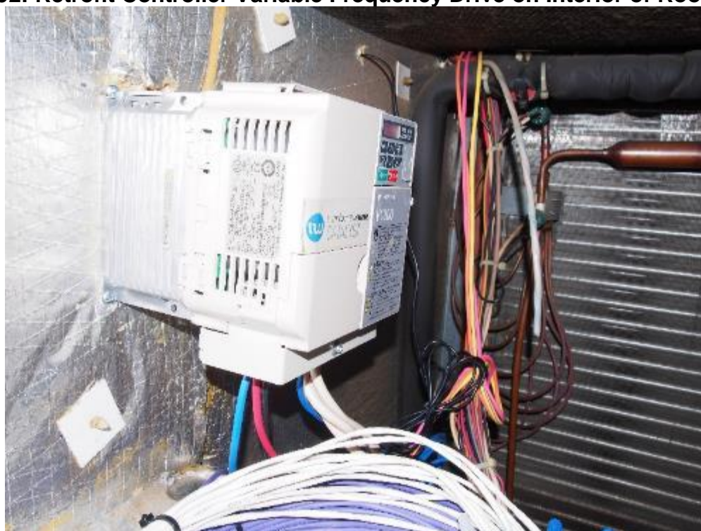
Figure 92: Retrofit Controller Variable Frequency Drive on Interior of Rooftop Unit
