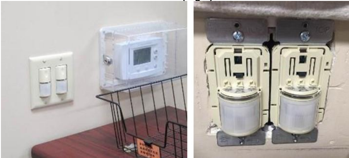
Figure 114: Wall Switch Occupancy Sensors (Left) and Exposed Programming Interface (Right)
