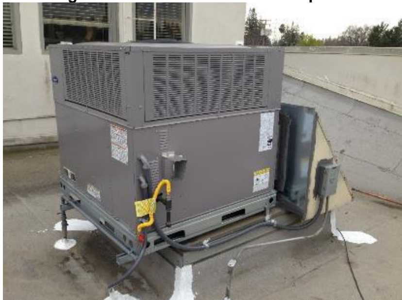
Figure 113: Post-Retrofit of Rooftop Unit
