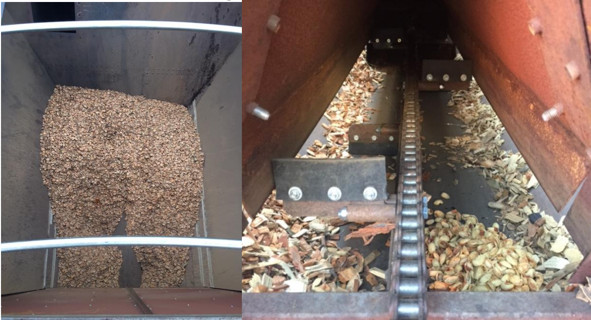
Figure 27: Hopper Feed System
