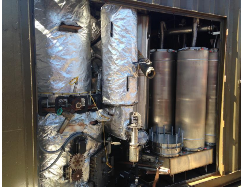
Figure 29: Gasifier and Filter
