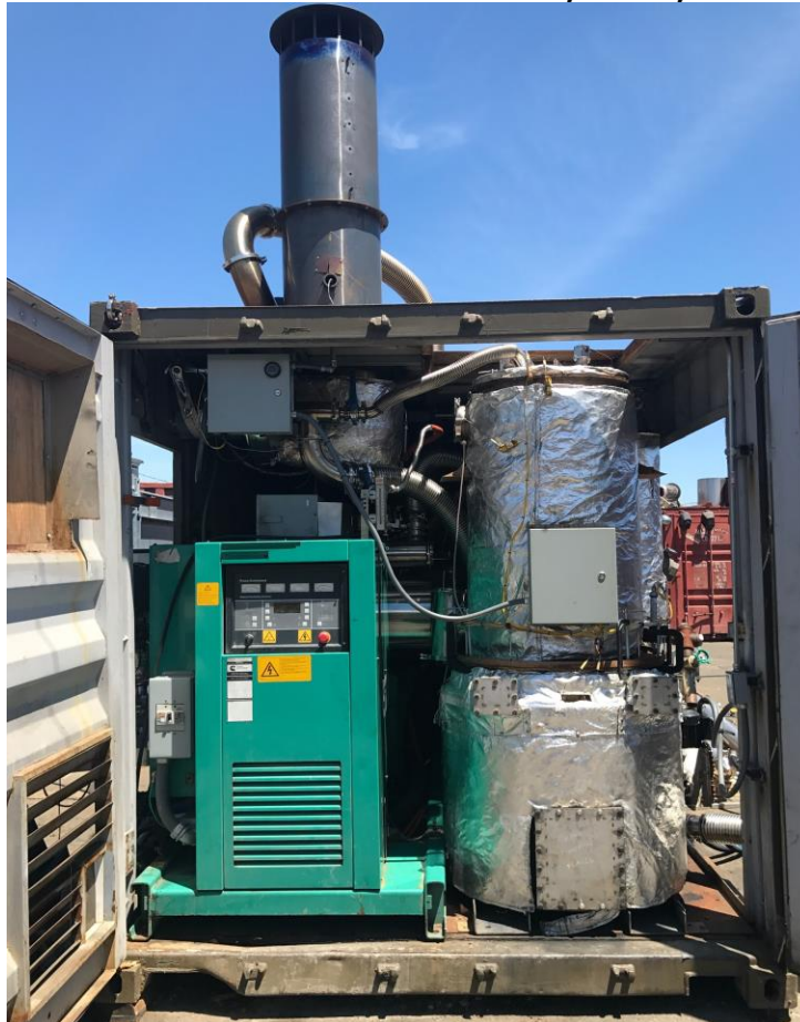
Figure 25: Powertainer with Gasifier, Flare, and Genset
