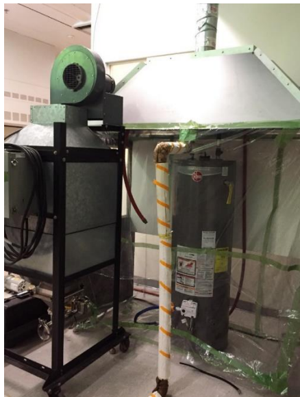
Figure 25: Water Heater Exhaust Sampling Setup
