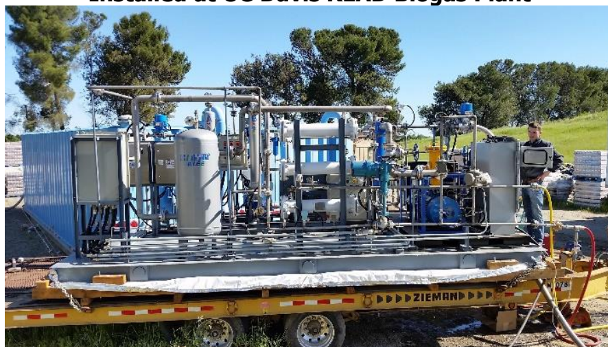
Figure 1: Helee LLC Upgrading Unit on Transportable Trailer Installed at UC Davis READ Biogas Plant
