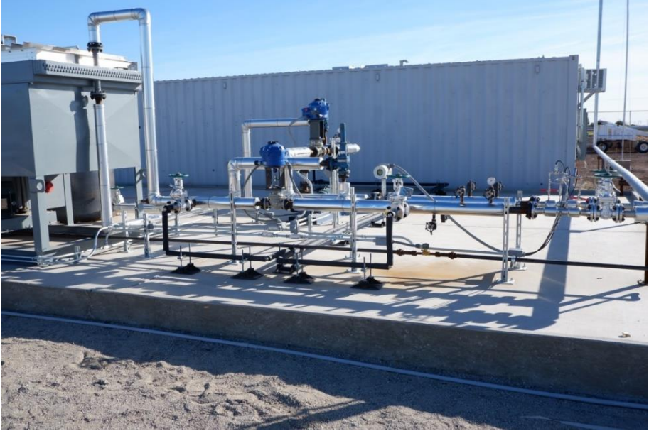
Hydrothermal processing and concentrating solar power system integration.
