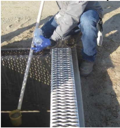
Figure 7: ABEC #3 Effluent Overflow Sump and Sampling Point
