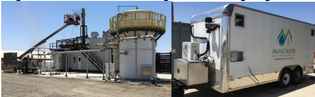
Figure 12: Stack Emission Testing at ABEC #3 Engine-generator
