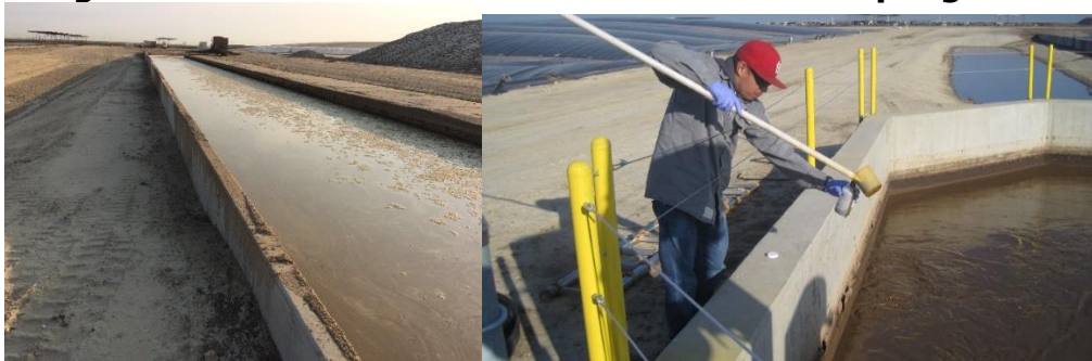
Figure 6: ABEC #3 Sand Lane and Influent Sampling Point
