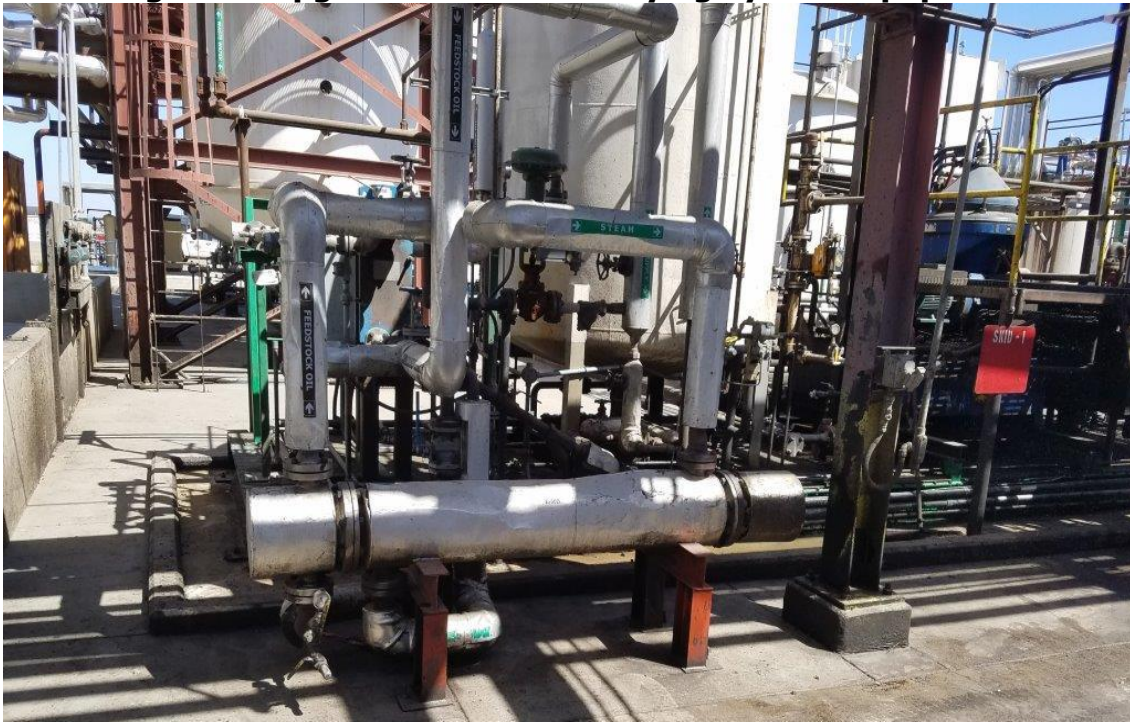
Figure 5: Upgraded Feedstock Drying System Equipment
