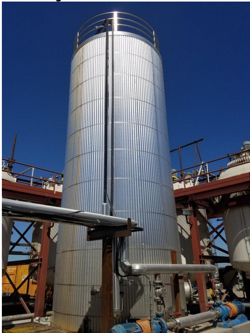
Figure 7: Installed Buffer Vessel
