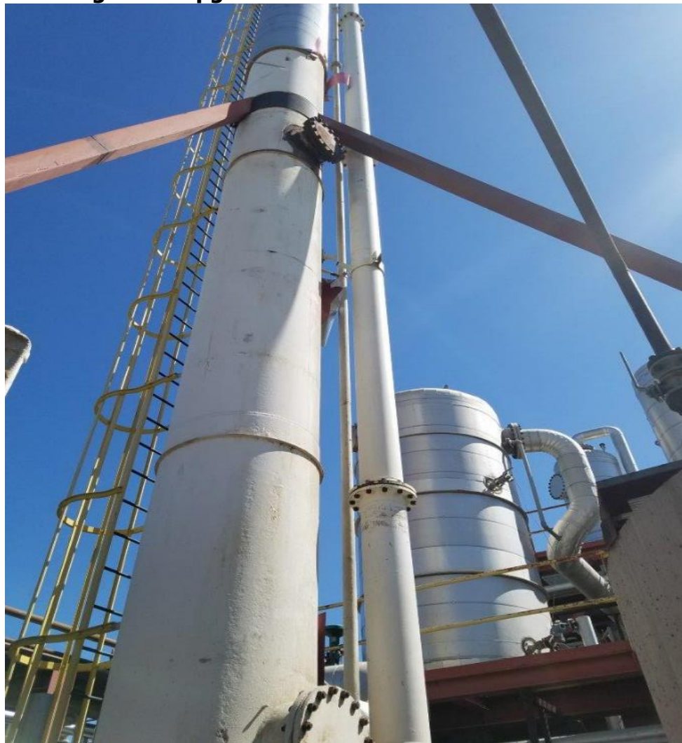
Figure 6: Upgraded Methanol Distillation Column
