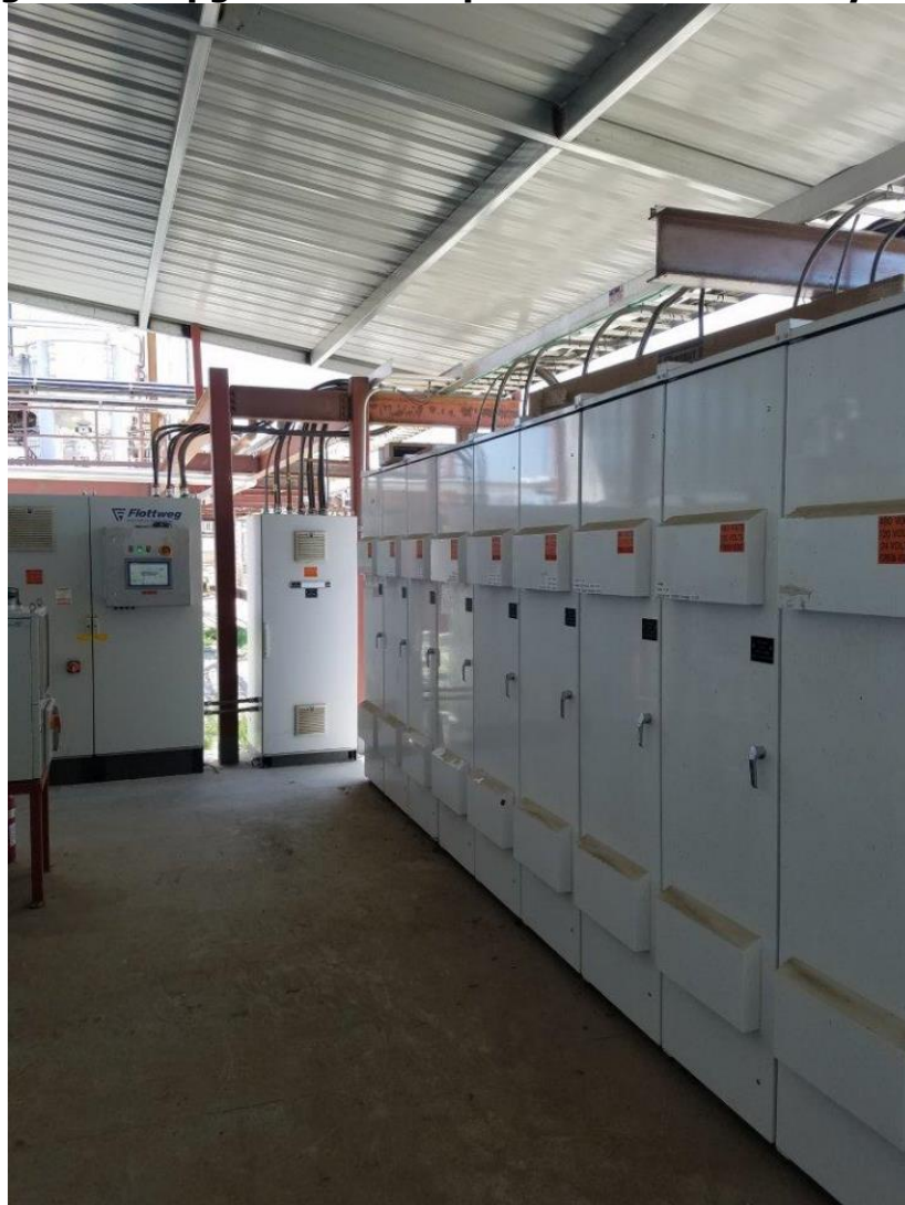
Figure 11: Upgraded and Expanded Automation System
