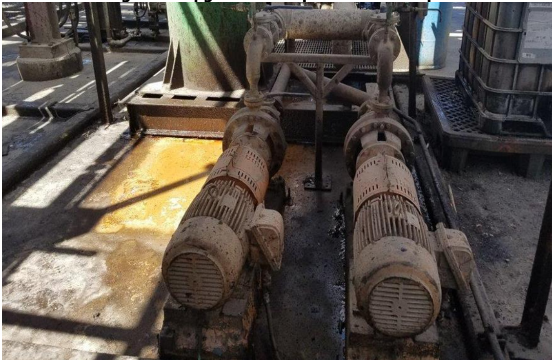
Figure 4: Upgraded 25 h.p. Transfer Pumps.
