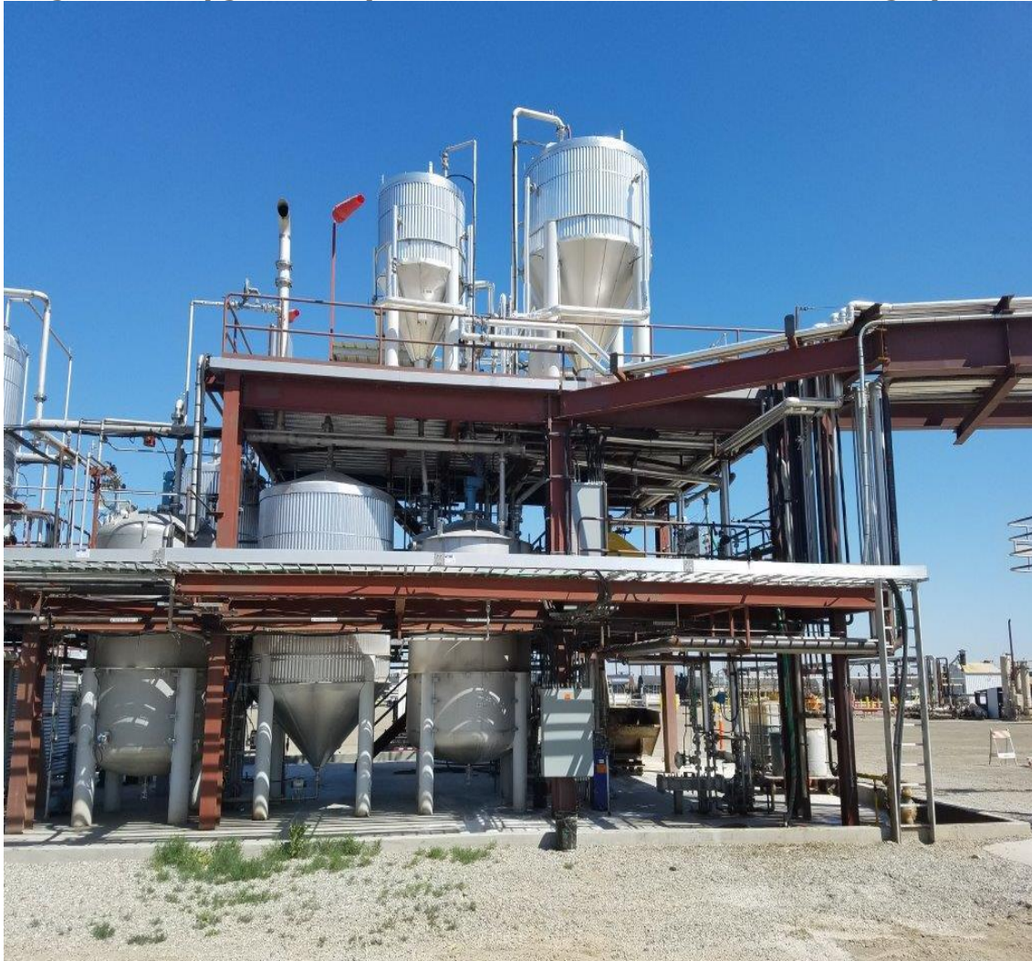
Figure 10: Upgraded Glycerin Neutralization and Processing System
