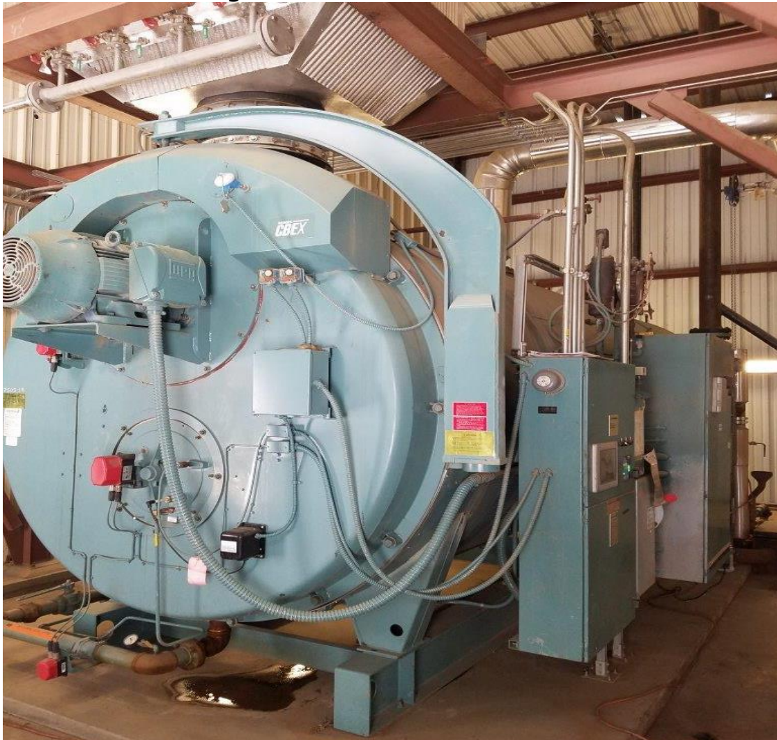
Figure 10: New Steam Generator
