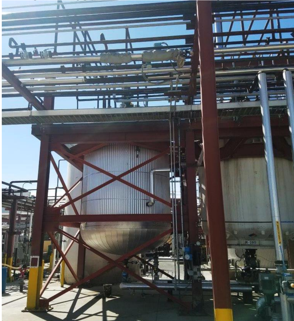
Figure 8: Upgraded Transesterification System Tank.
