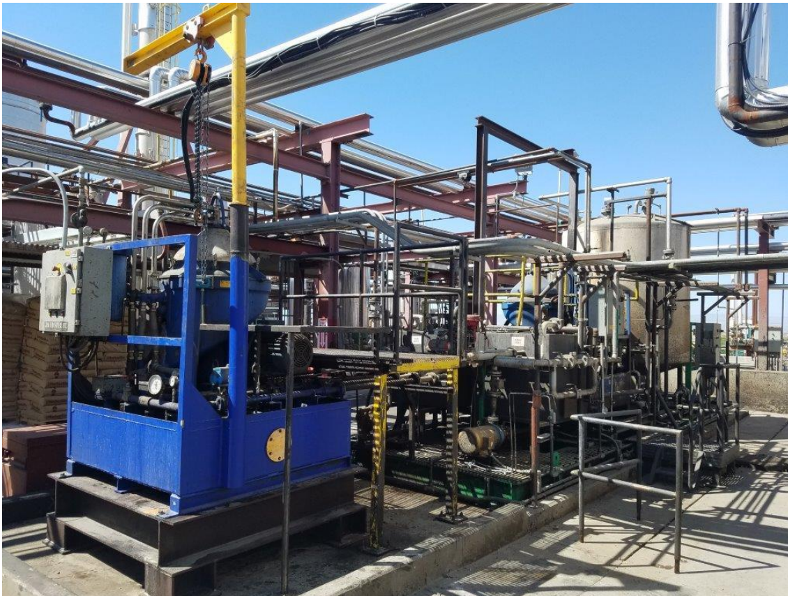
Figure 3: Upgraded Decanting Centrifuge
