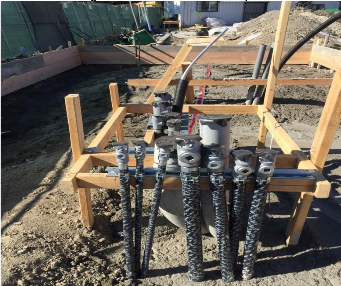
Figure 4: Station Conduit "Stub-ups"
