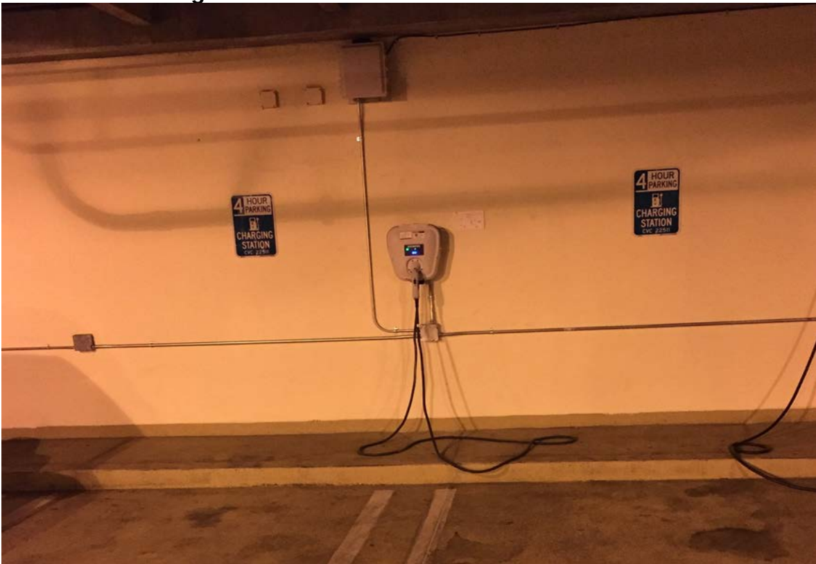
Figure 8: Installation at LADOT: Robertson
