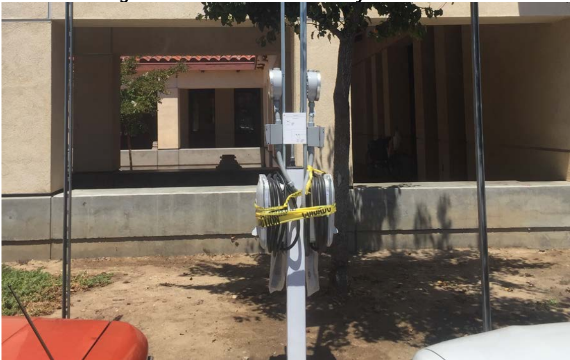
Figure 20: Installation at Library: Chatsworth
