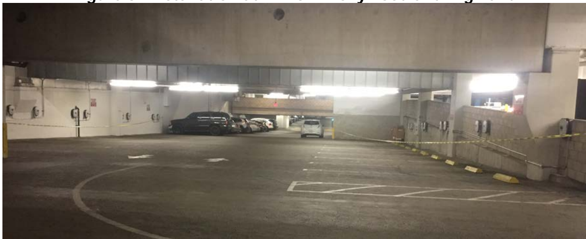
Figure 5: Installation at LADOT: Hollywood and Highland
