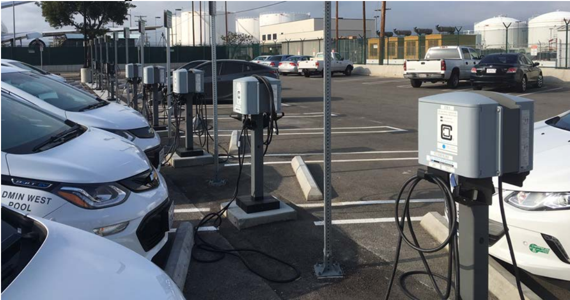
Figure 16: Installation at LAWA: Admin West
