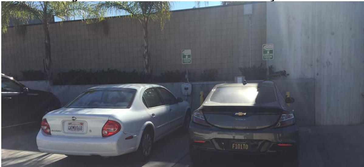
Figure 13: Installation at LAPD: North Hollywood
