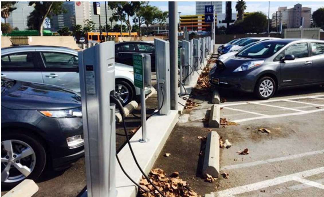
Figure 17: Installation at LAWA: Parking Lot C
