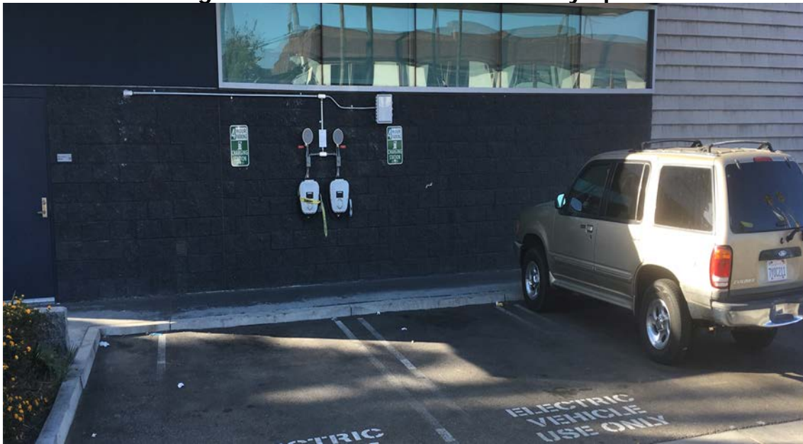
Figure 14: Installation at LAPD: Olympic
