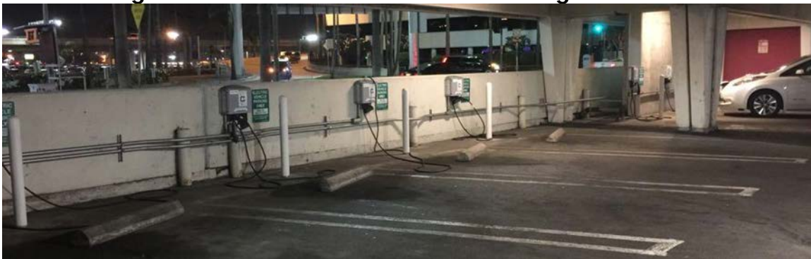
Figure 19: Installation at LAWA: Parking Structure 7
