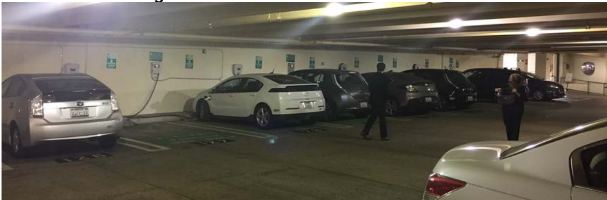
Figure 3: Installation at LADOT: Broxton
