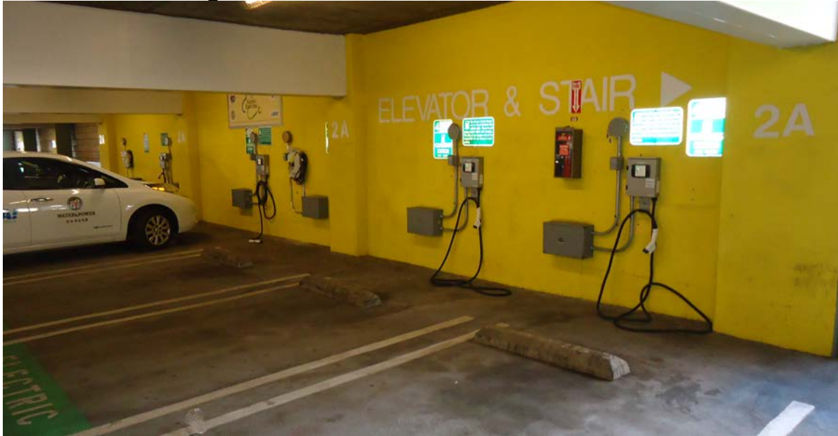
Figure 4: Installation at LADOT: Cherokee
