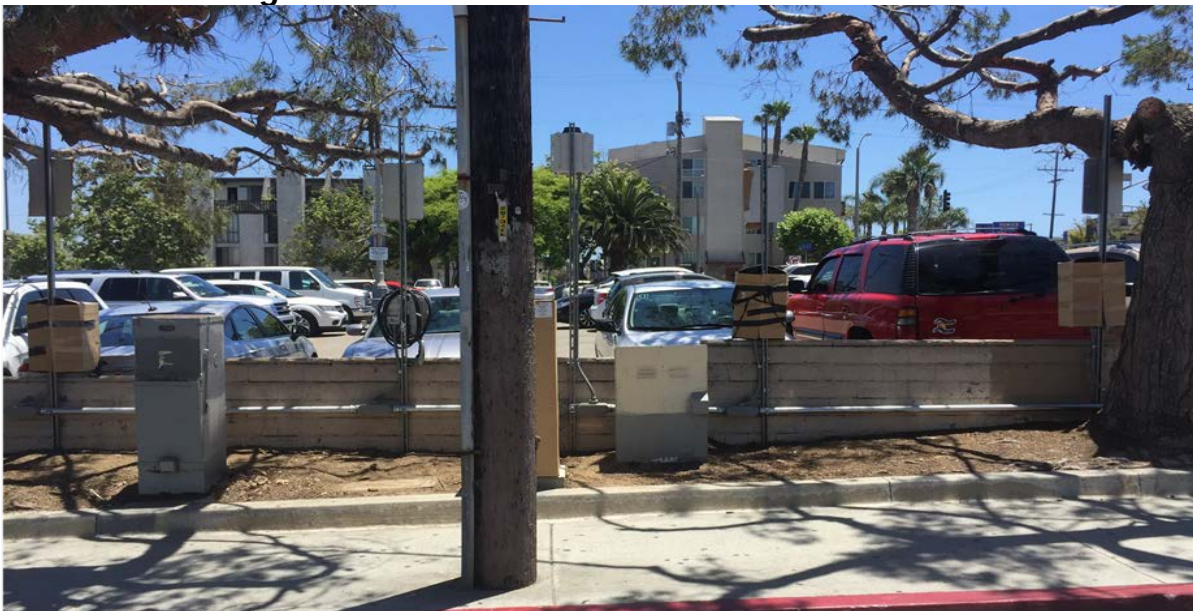
Figure 9: Installation at LADOT: Venice Beach
