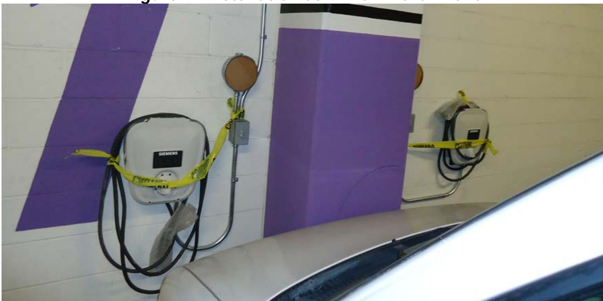
Figure 7: Installation at LADOT: Larchmont
