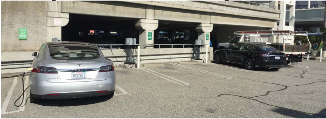
Figure 18: Installation at LAWA: Parking Structure 1
