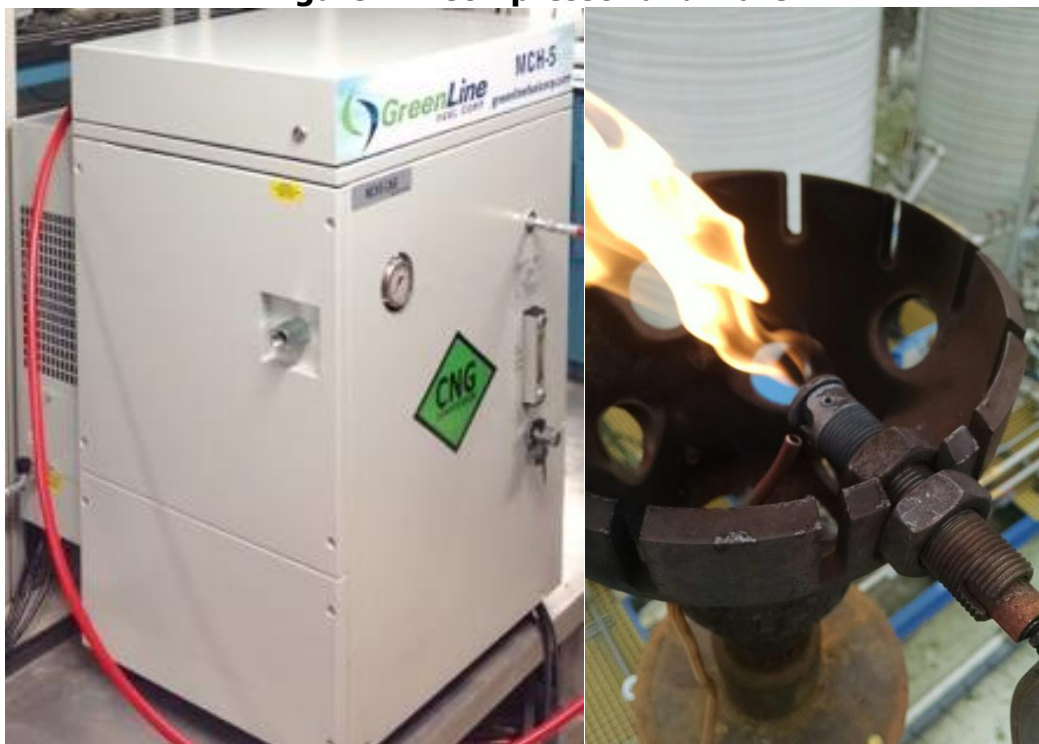
Figure 24: Compressor and Flare
