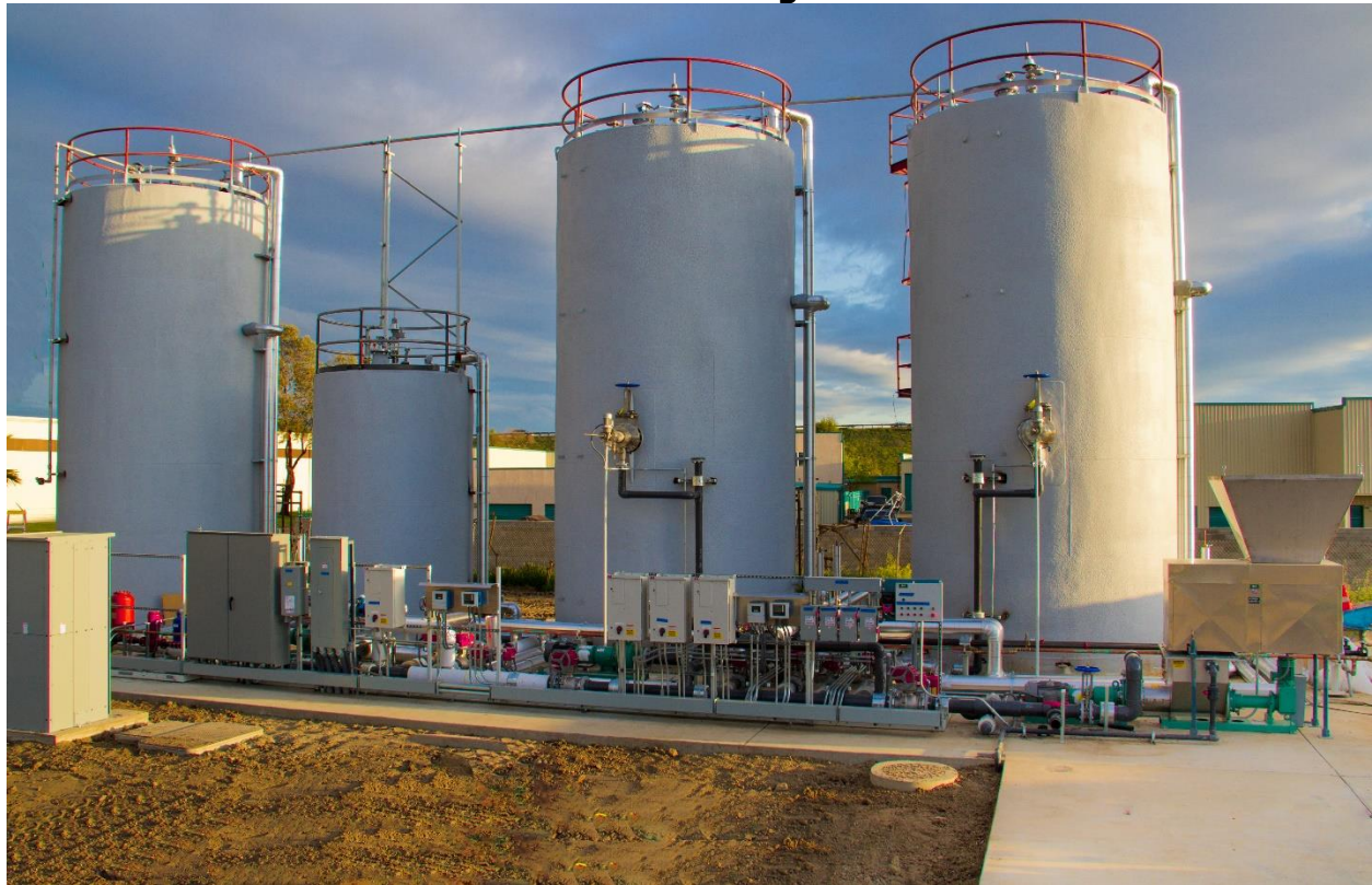
Figure 25: Nominal 100,000 Gallon CleanWorld High Rate Digester System Used for Pilot Testing
