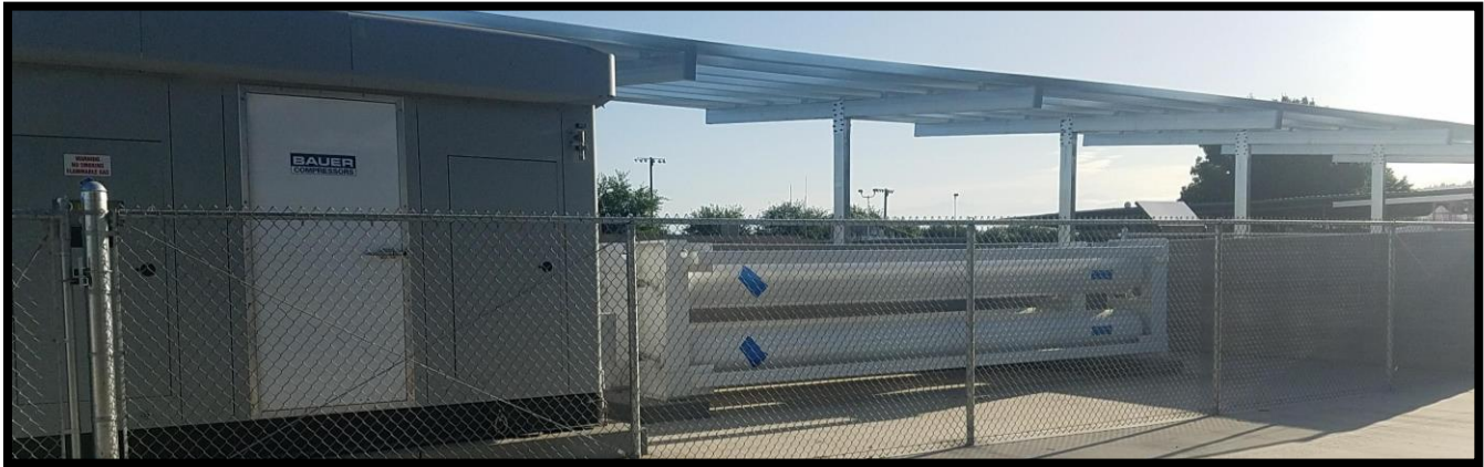
Figure B-1: Bauer CNG Compressor Package and CP Industries CNG Storage Vessels
