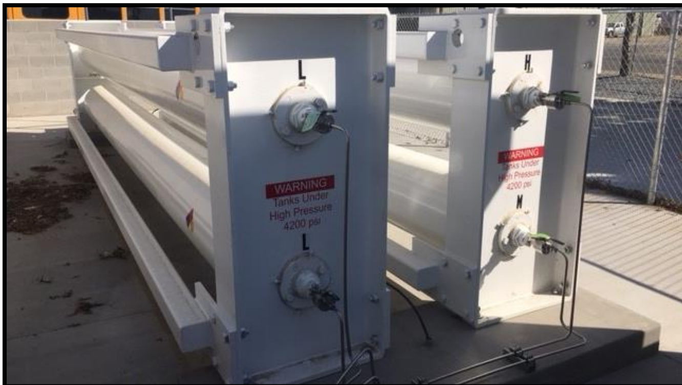
Figure B-5: CP Industries CNG Storage Vessels
