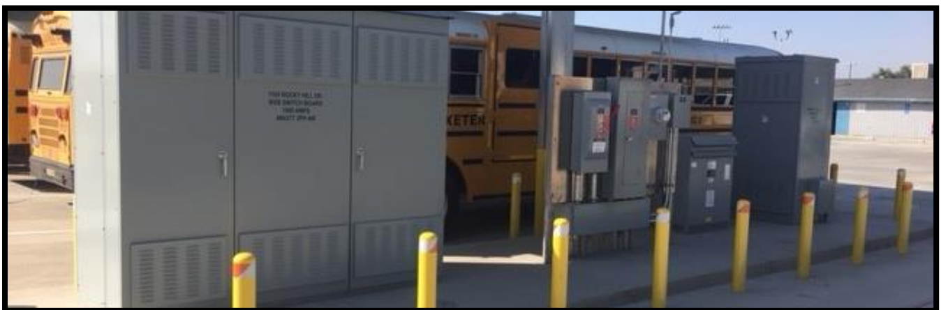
Figure 4: Upgraded Electrical Service
