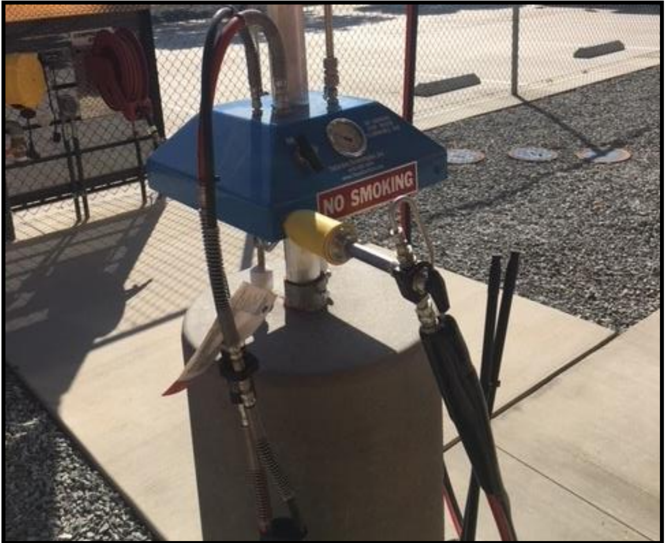
Figure B-11: Broadlux/Com Data Fuel Management System
