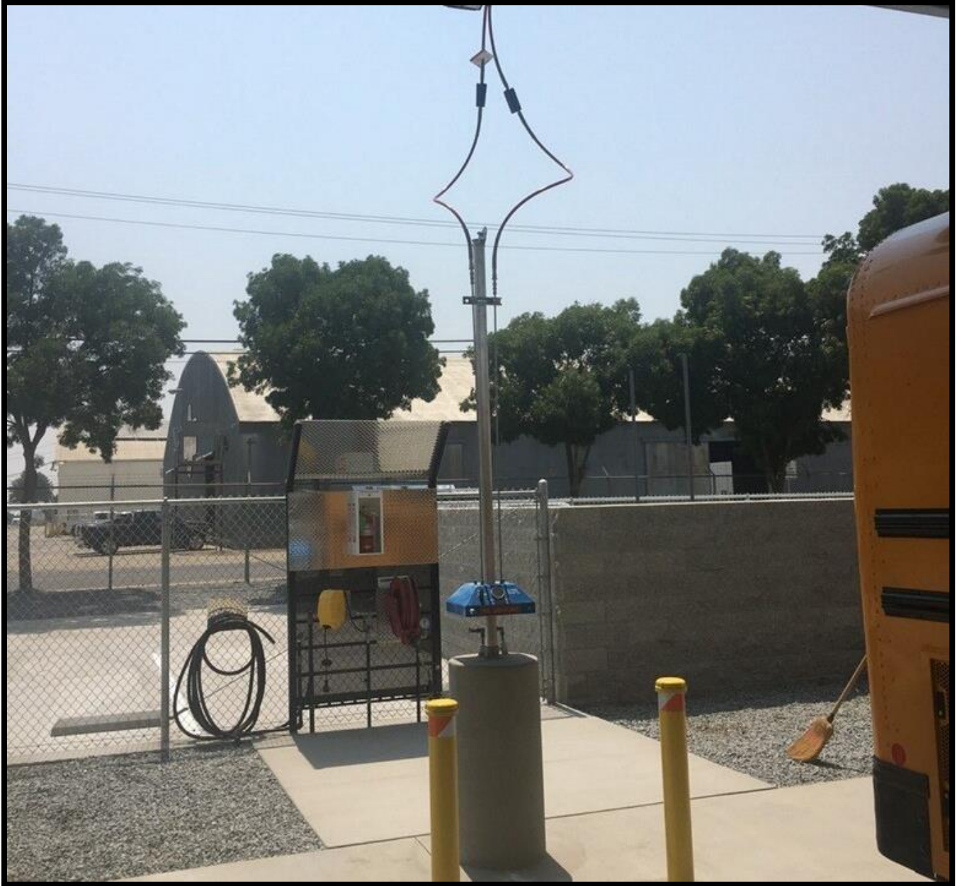
Figure B-10: Broadlux/Com Data Fuel Management System
