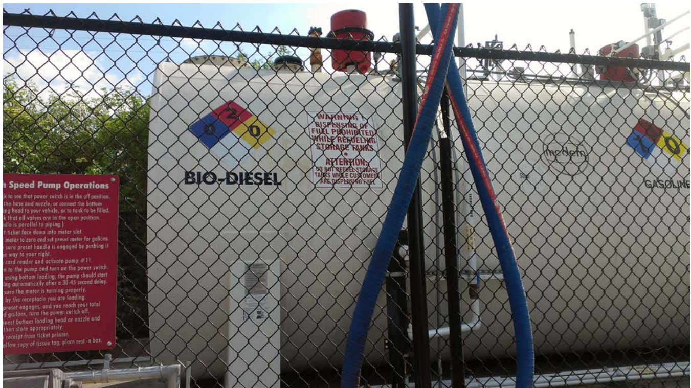
Figure 3: Biodiesel-Diesel Split Storage Tank
