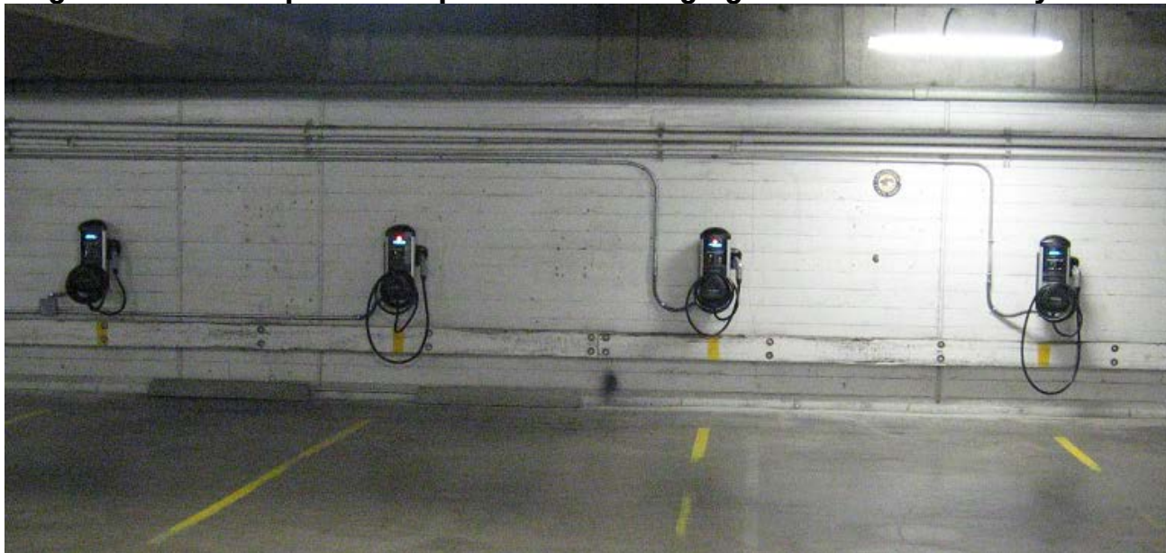
Figure 4: Dual Purpose Workplace/Fleet Charging Stations w/Card Key Access
