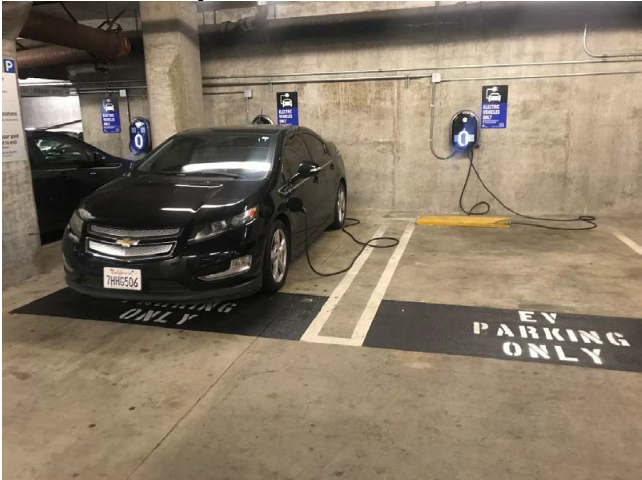
Figure 6: Union Station Installation
