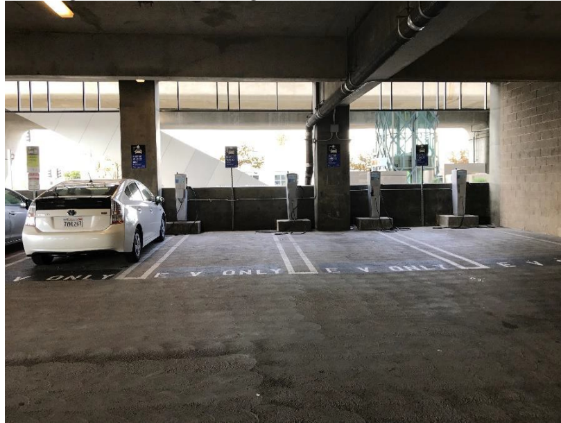
Figure 3: La Cienega/Jefferson Installation
