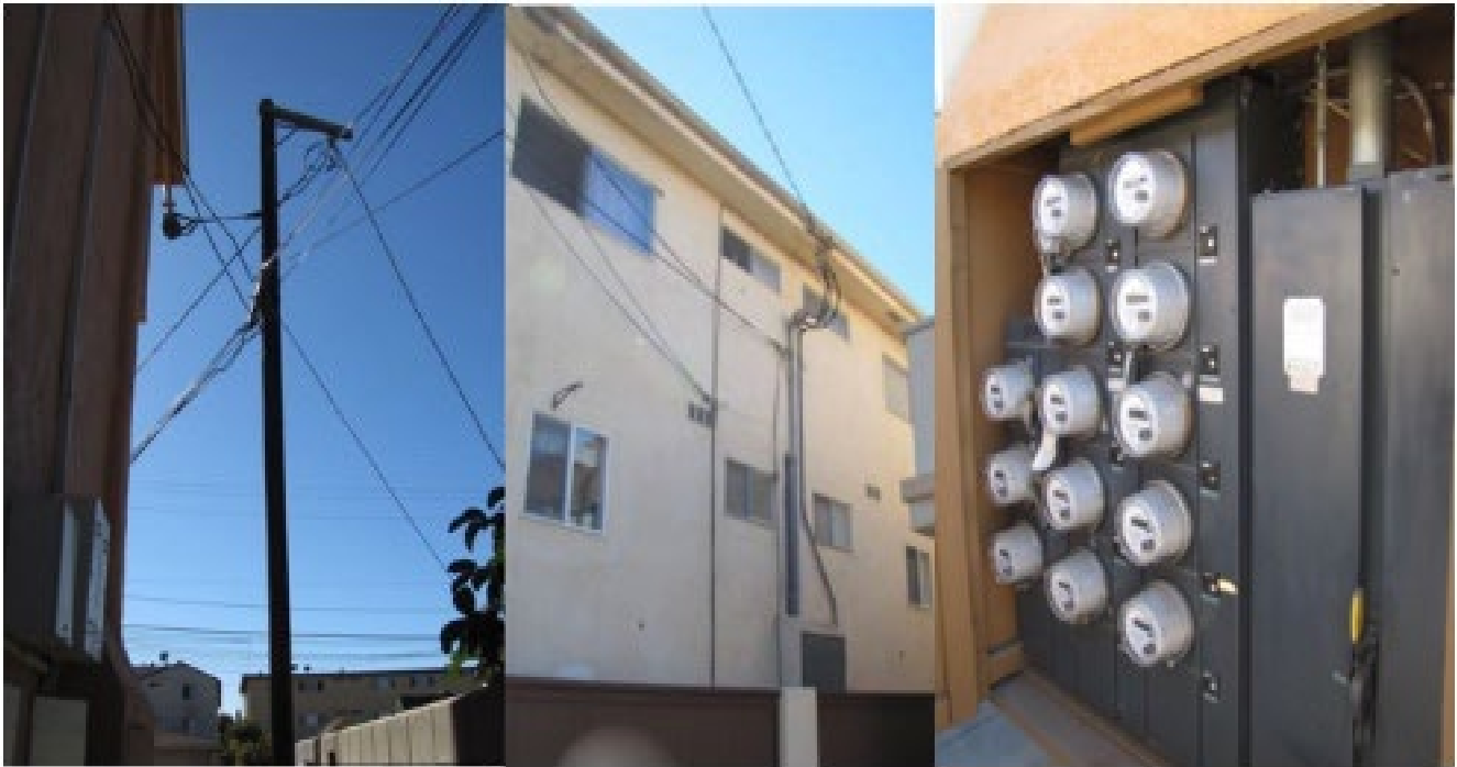
Figure 12: Photos of Overhead Service Drops and Meters at MUDs
