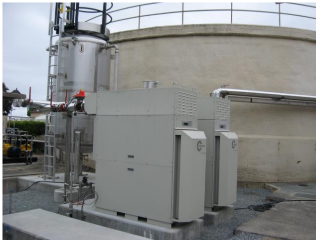
Figure 5: View of the Two Capstone Microturbines With a Third Foundation for Future Installation
