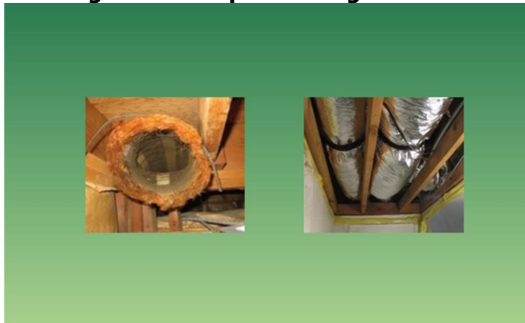
Figure 19: Proper Ducting Installed
