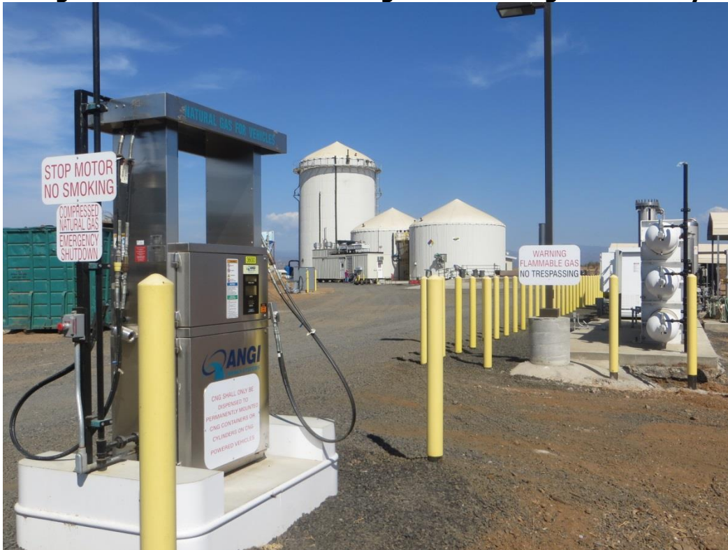
Facility with refueling station (foreground) and digesters (background) from PIR-14-022 project.
