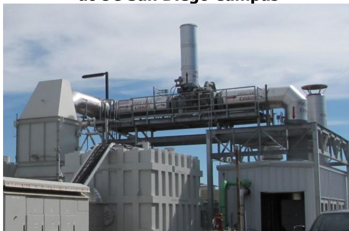
Figure 5: 2.8 MW Fuel Cell Integrated with Absorption Chiller at UC San Diego Campus
