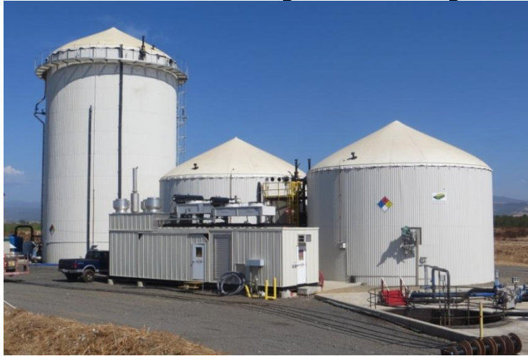
Figure 4: North State Rendering Anaerobic Digester Facility
