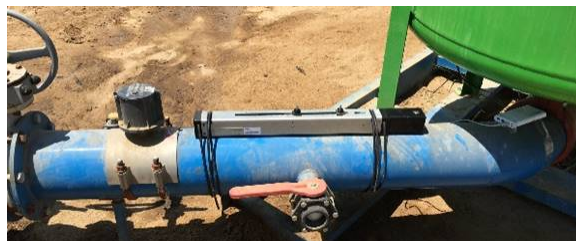
Figure A-2. Daily water measurement performed with jWave acoustic meter from Seametrics.
