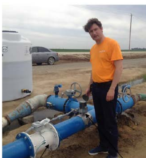
Pump 19 (VFD controller)
