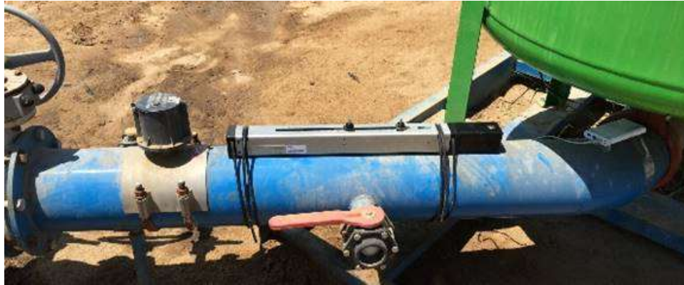
Figure 19: Acoustic Meters Temporarily Installed at One Pumping Station During the Project
