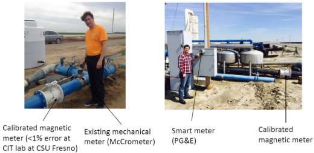
Figure 18: Magnetic Meters Installed at Two Pumping Stations at Site #6 in Helm, California
