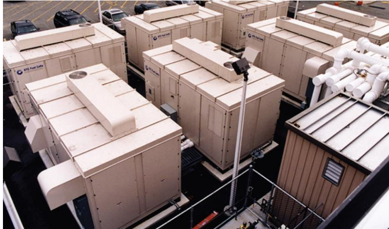
Figure 9: CHP Fuel Cell Installation at Verizon Data Center
