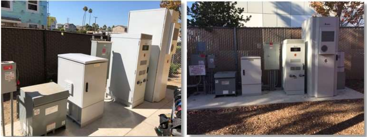
Figure 7: Fire Station 6 and 7 Modular, Outdoor Microgrid
