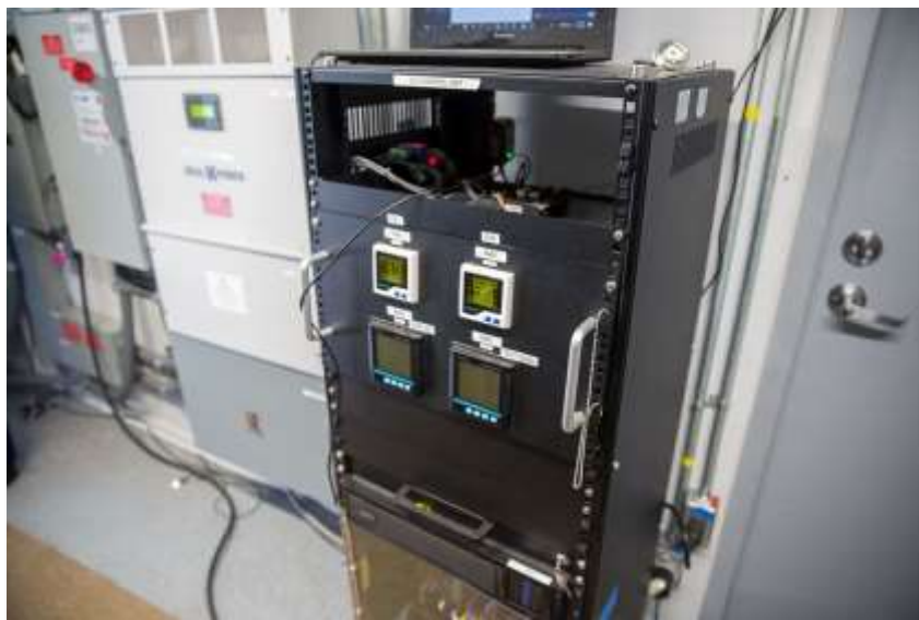
Figure 18: First Generation EnergyScope™ Microgrid Controller, Fire Station 11
