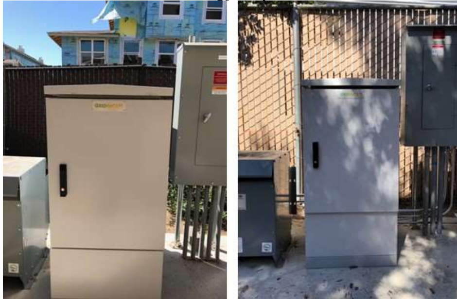
Figure 19: Second Generation EnergyScope™ Controller, Fire Station 6 & 7
