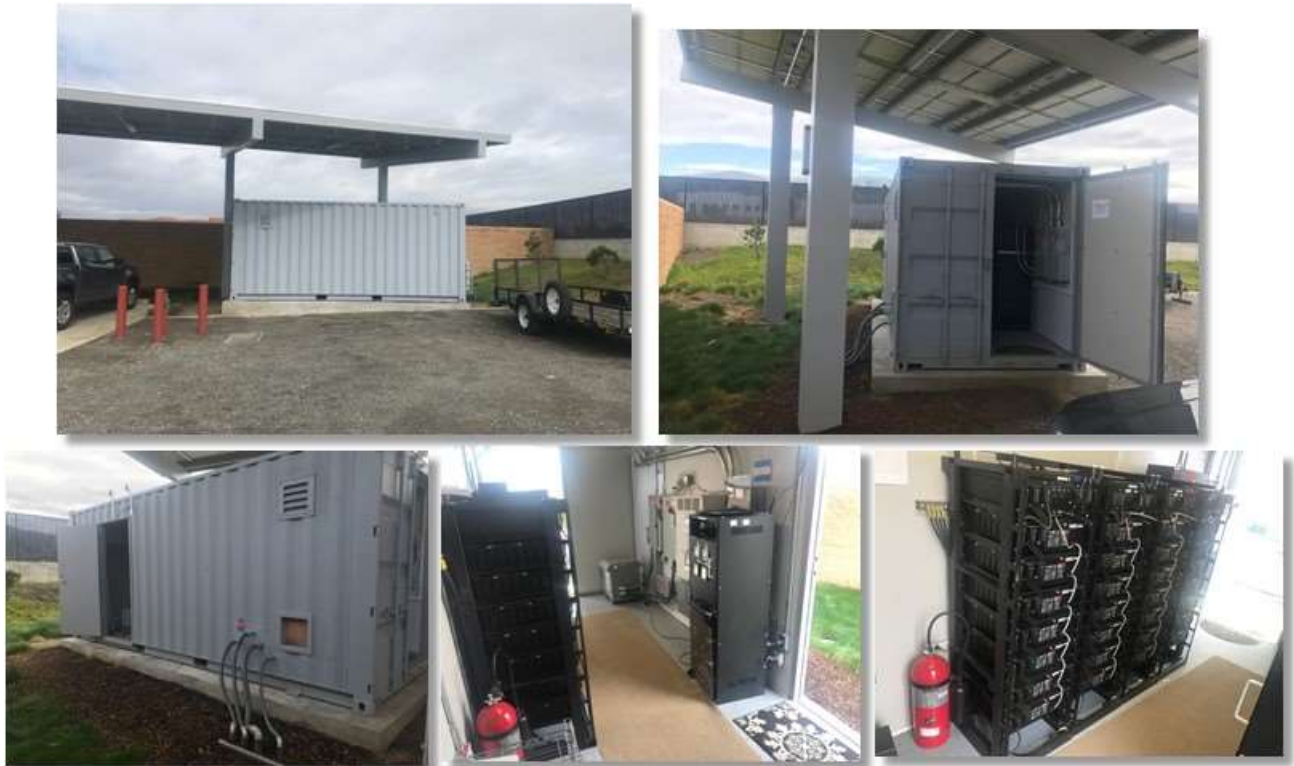
Figure 6: Fire Station 11 Microgrid Container Design
