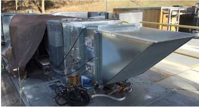
Figure B-3: Ebtron Gold Probes Installed with Two Different Air Intake Hoods
