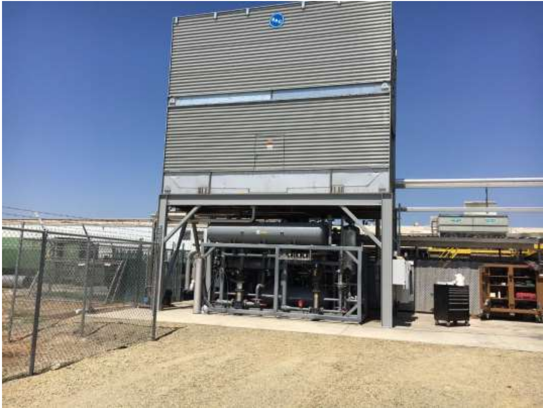
The ThermoSorber with cooling tower stacked on top.
