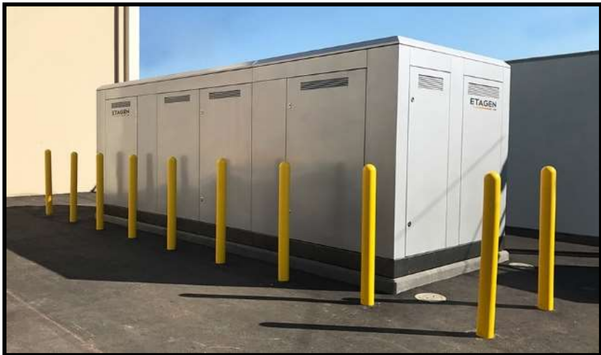
Figure 9: Enclosed Installation of Etagen Linear Generator Combined Heat and Power System
