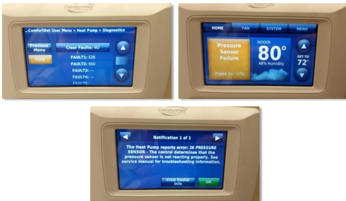
Figure 72: Thermostat Displays with Pressure Sensor Fault
