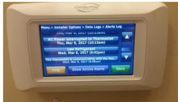
Figure 88: Thermostat Display of Low Refrigerant Fault on Alerts Log
