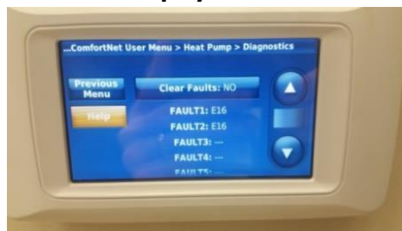
Figure 77: Thermostat Display with Minor Low Pressure Fault
