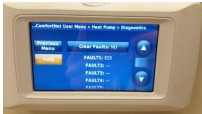
Figure 70: Thermostat Heat Pump Diagnostics Page with Air Sensor Fault
