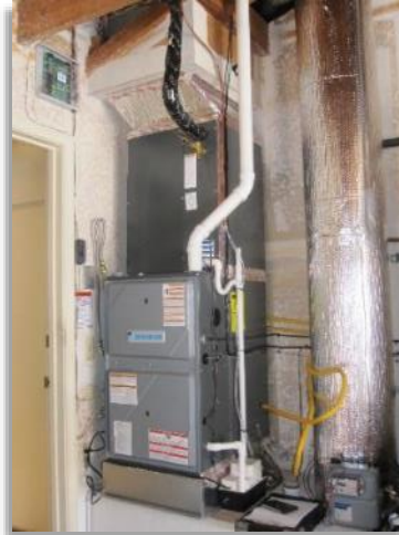
Figure 126: Vertical Configuration of Indoor Unit and Furnace in SDG&E Host Site Garage
