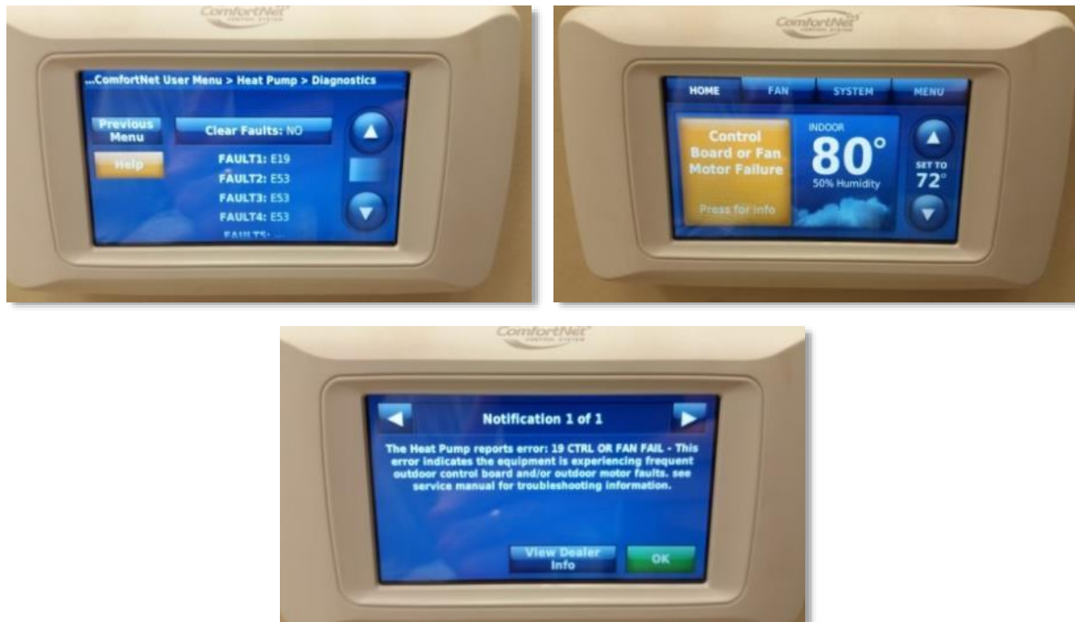
Figure 73: Thermostat Displays with Faults from Outdoor Fan Blockage
