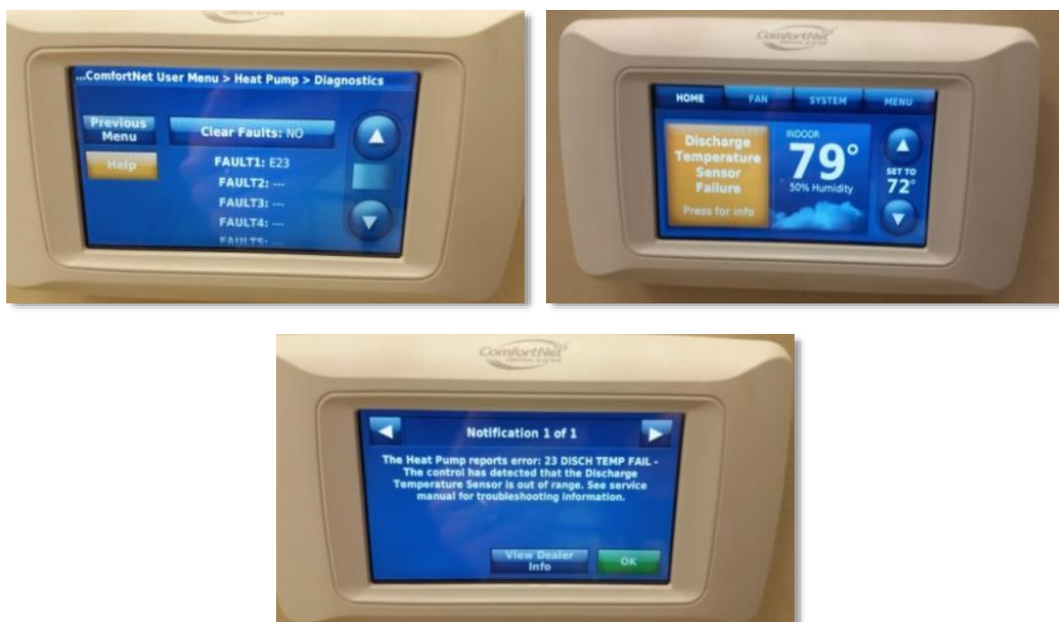
Figure 71: Thermostat Displays with Discharge Temperature Sensor Fault
