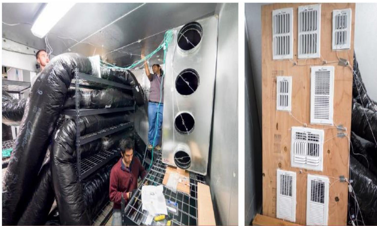
Figure 46: Duct and Grille Layout in WCEC Outdoor Environmental Chamber
