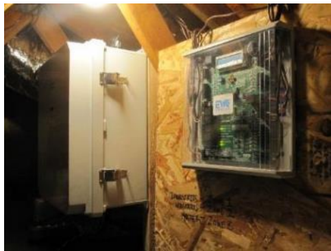
Figure 124: EPRI M&V Data Monitoring Box and EWC Zonal Control Board in Attic at SCE Host Site
