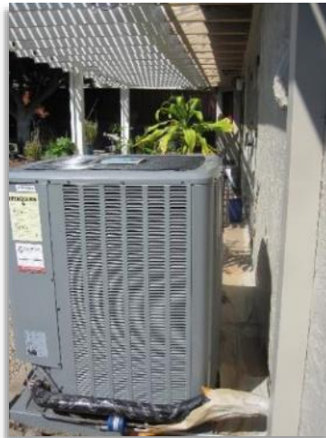
Figure 127: Next-Gen RSCS Outdoor Unit at SDG&E Host Site Backyard
