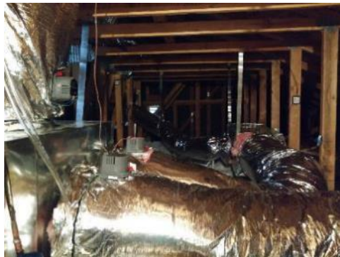
Figure 122: PG&E Host Site Attic with Horizontal Configuration of Indoor Unit and Furnace
