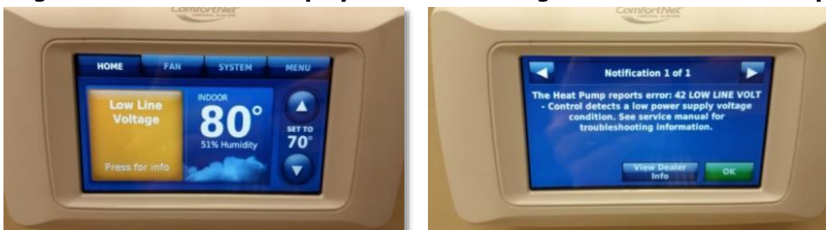
Figure 75: Thermostat Displays with Low Voltage Fault at the Heat Pump
