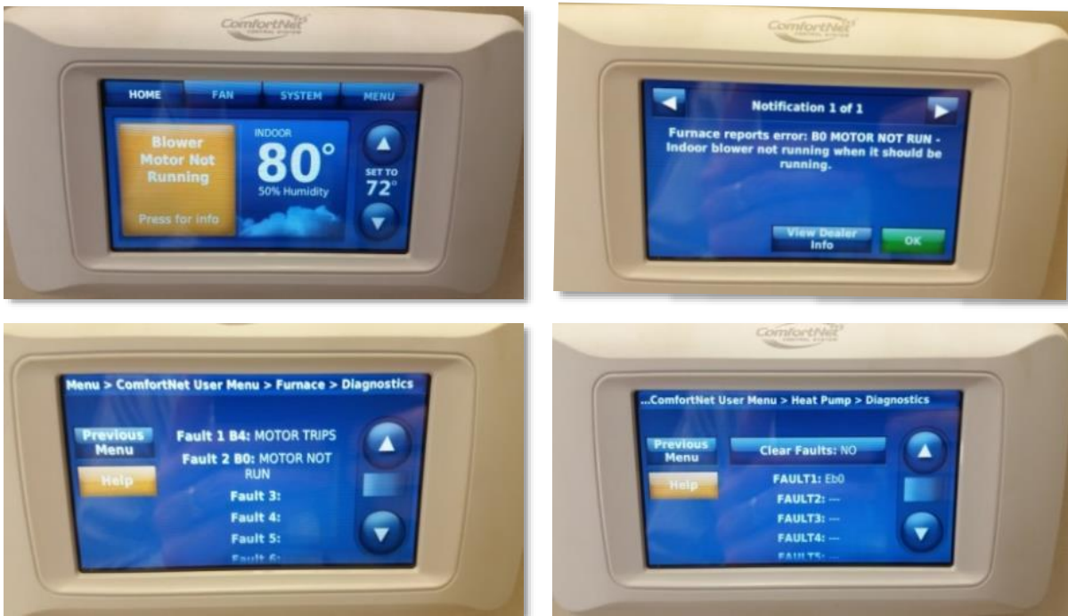
Figure 74: Thermostat Displays with Faults from Indoor Blower Blockage
