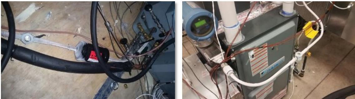
Figure 76: Frosting of Liquid Line with Service Valve Almost Closed
