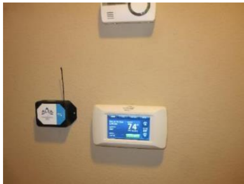
Figure 125: CTK04 Thermostat and Wireless Temperature/Relative Humidity Sensor at SCE Host Site
