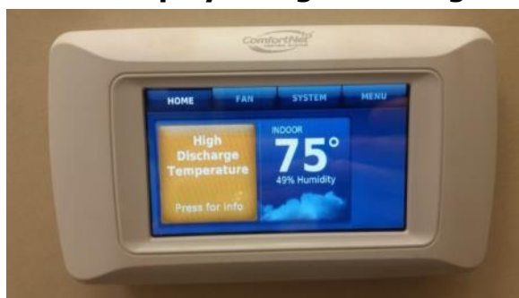
Figure 96: Thermostat Display of High Discharge Temperature Fault
