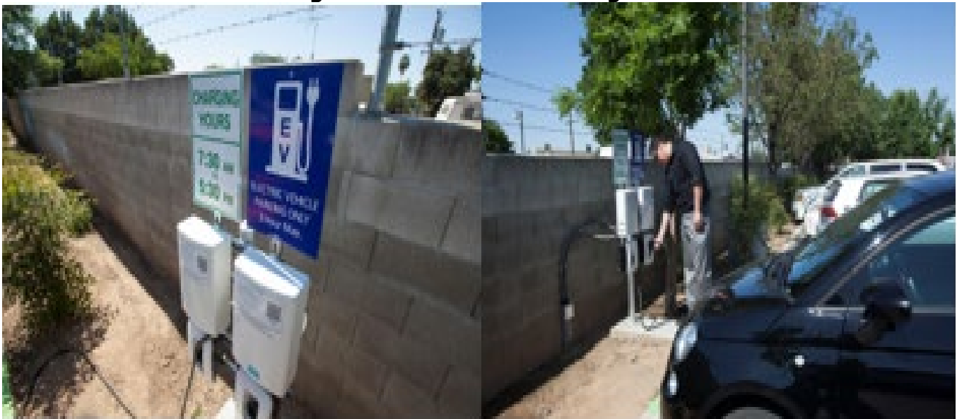
Figure 1: Fresno Office Chargers:
