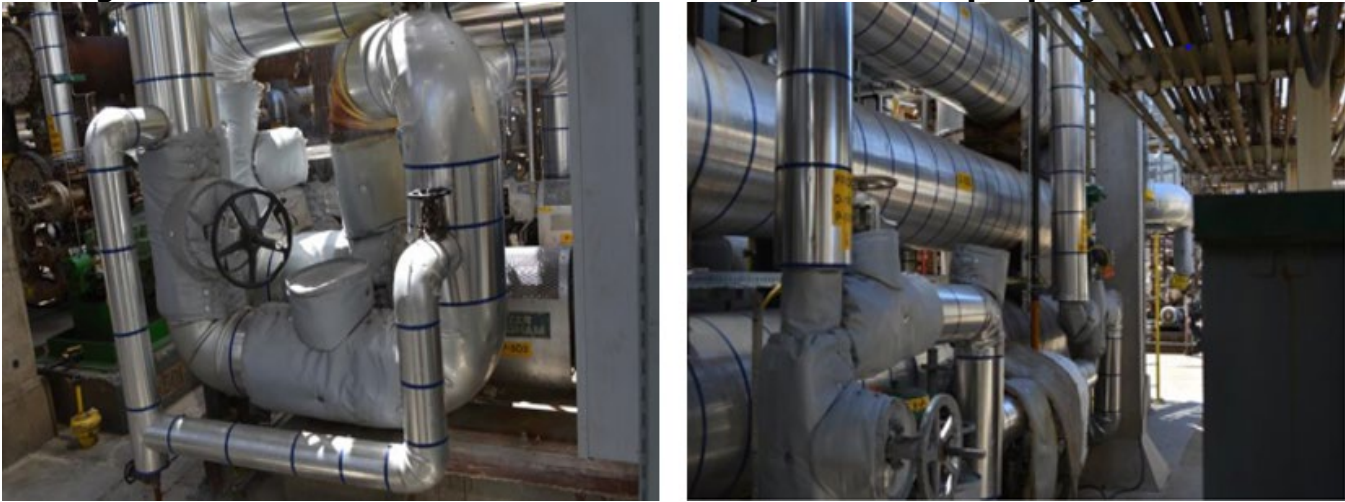
Figure 7: Installed Stainless Steel and Alloy Reactor Loop Piping and Valves
