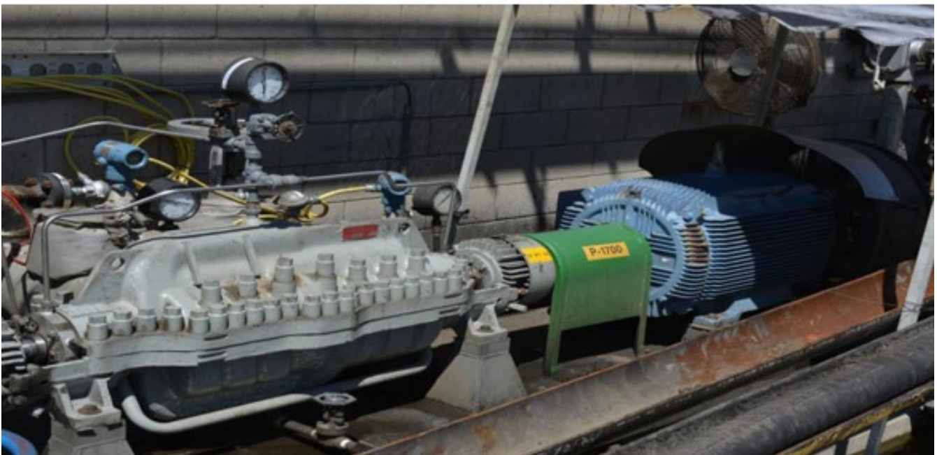
Note: Top: Fresh Hydrogen Compressor (C-122, above), Bottom: Tallow Feed Charge Pump (P-1700)
