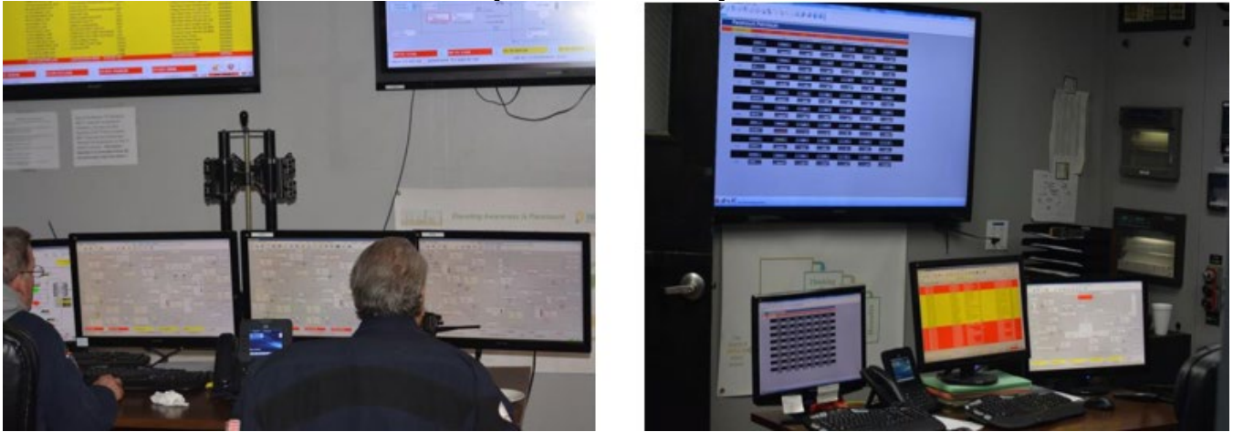
Figure 11: Migrated Existing Control Equipment into a New Control Room with New Computer Control System
