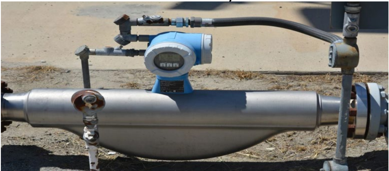
Figure 10: New and Reworked Meters and Associated Equipment to Make A State-Of-The-Art Control System
