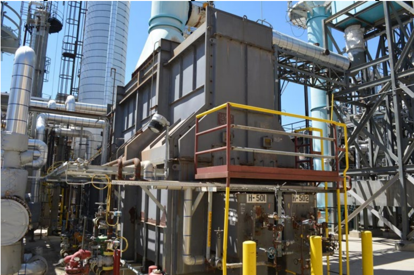
Figure 8: Retubed Reactor Charge Heaters with Stainless Steel Tubing
