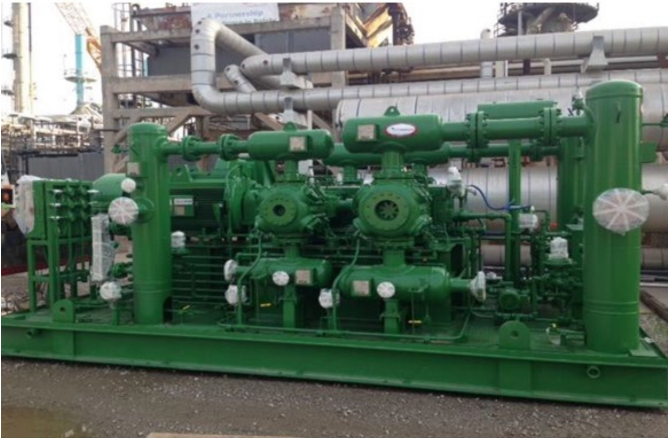
Figure 3: New Equipment Photos
