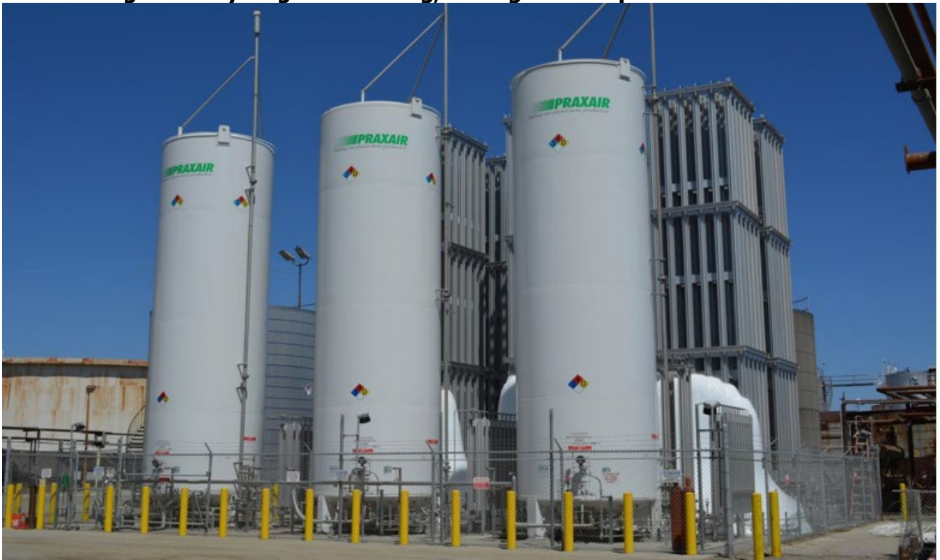
Figure 9: Hydrogen Receiving, Storage and Vaporization Facilities
