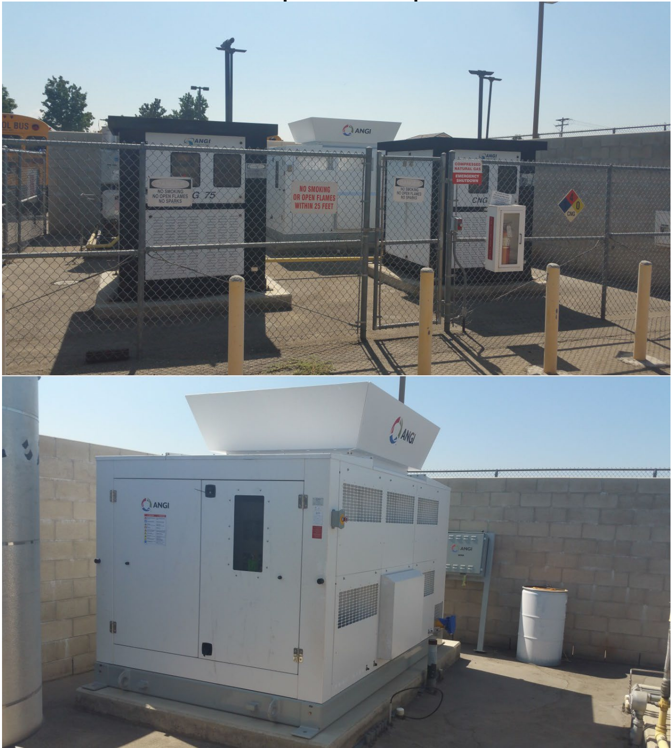
Figure 6: 75 standard cubic feet per minute Compressors and ANGI 225 standard cubic feet per minute Compressor
