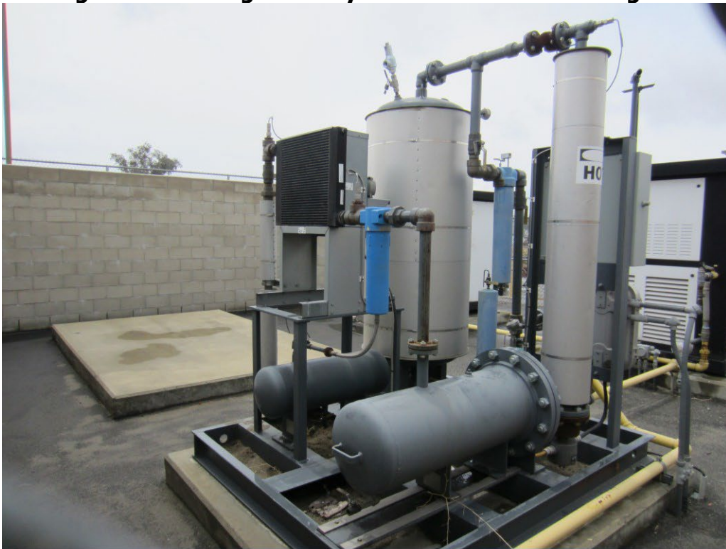
Figure 3: Existing CNG Dryer and Electrical Switchgear
