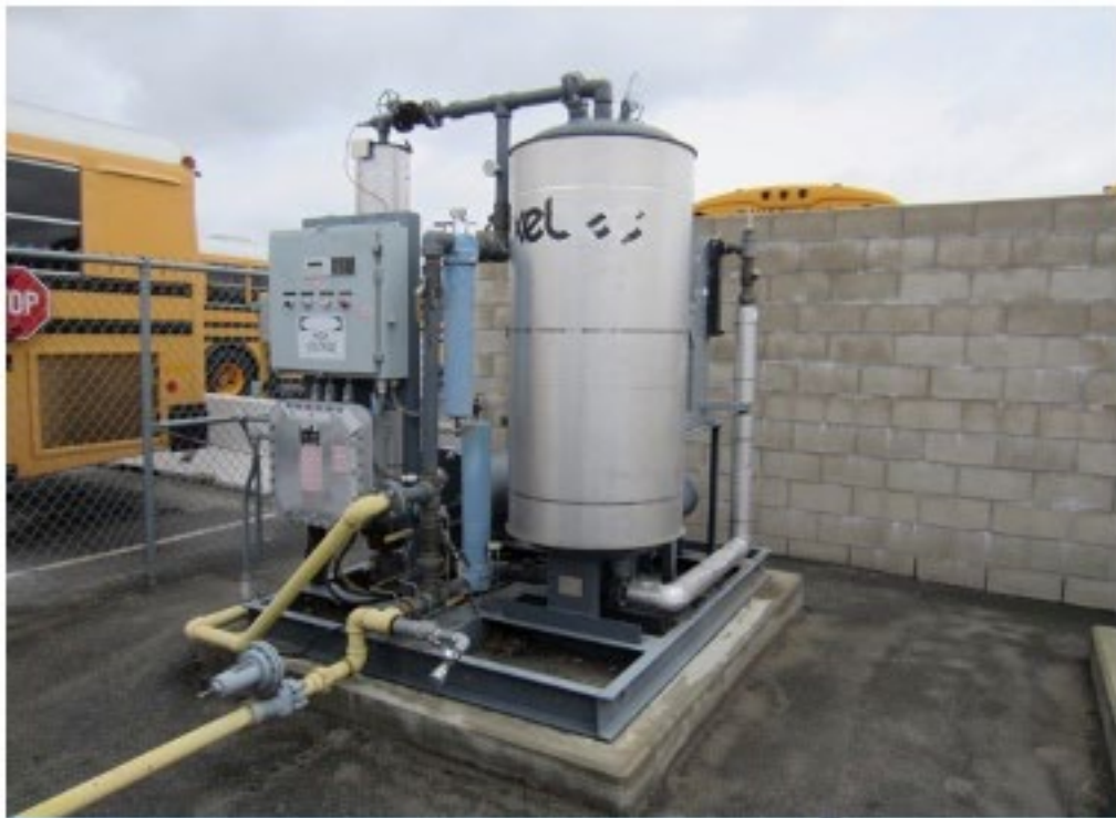
Figure 5: Front of Existing CNG Dryer and New Electrical Panel
