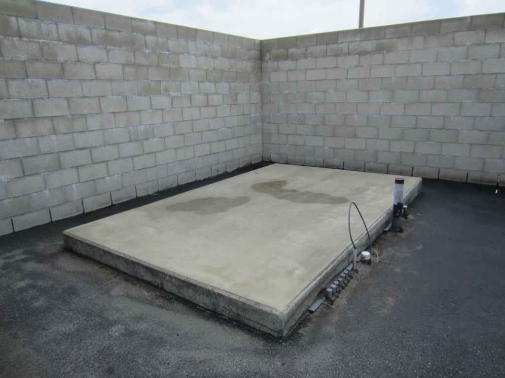
Figure 2: Concrete Slab and 2 75 standard cubic feet per minute Compressors
