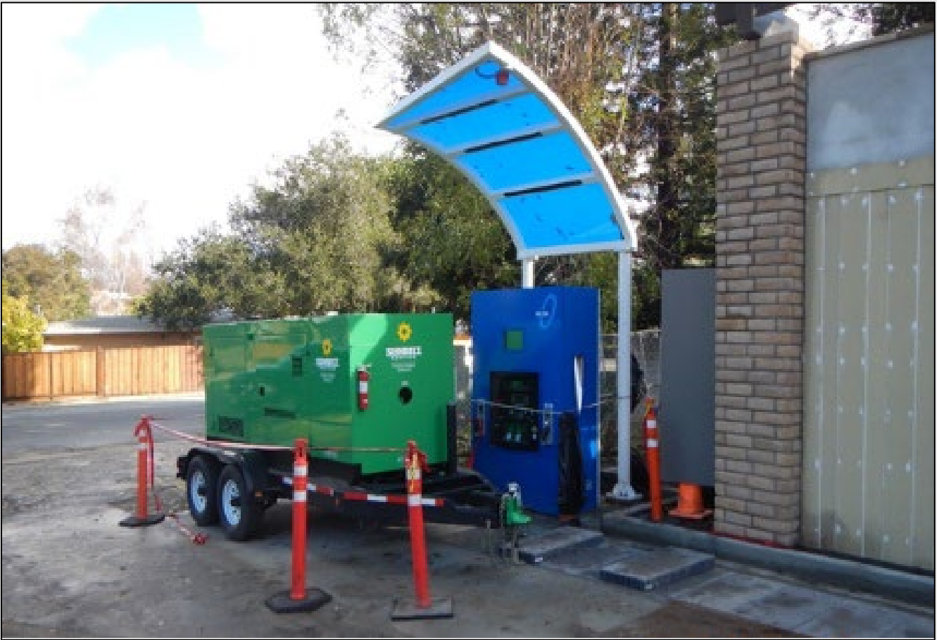
Figure 7: Generator During Station Commissioning
