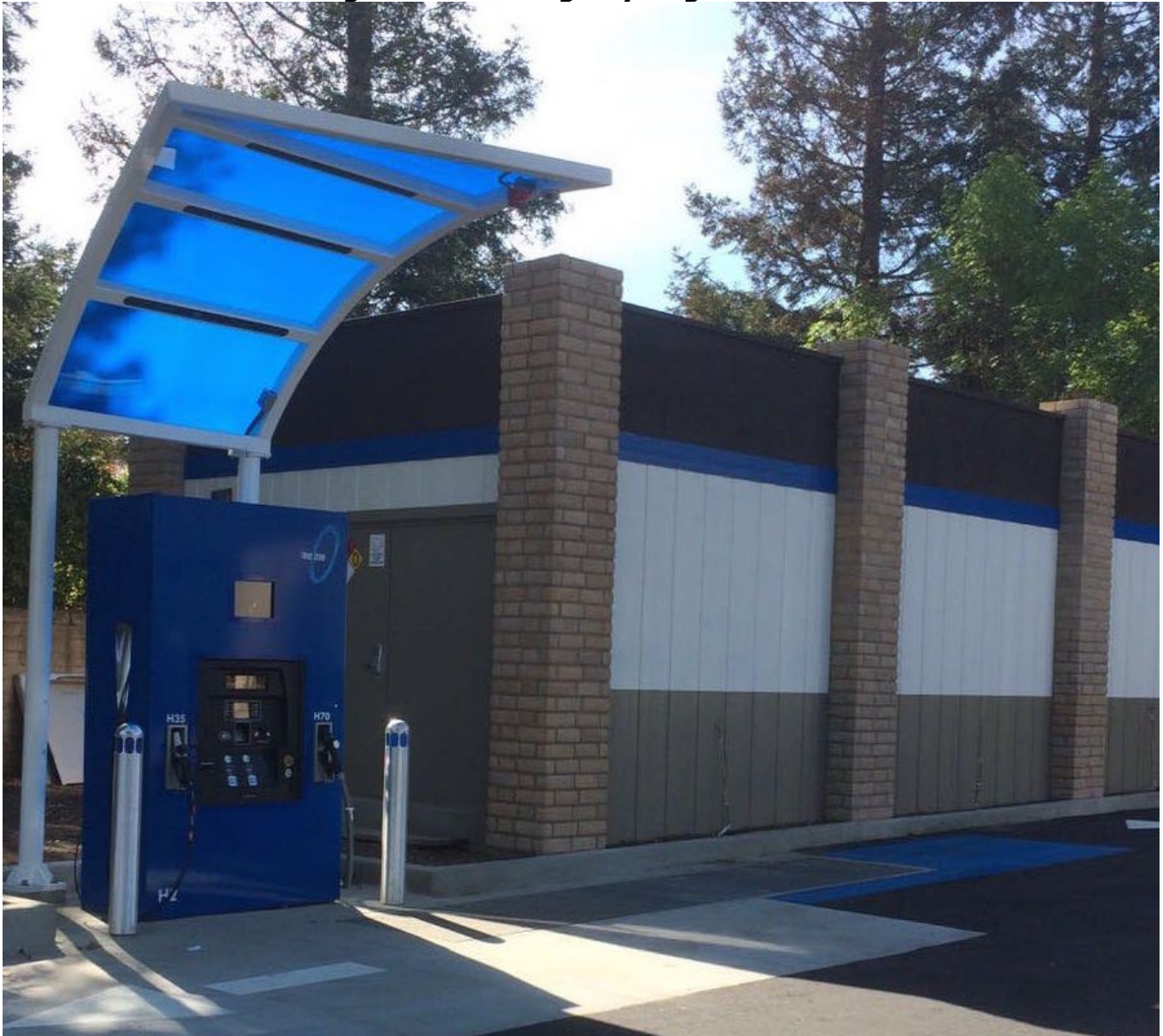
Figure 12: Saratoga Hydrogen Station
