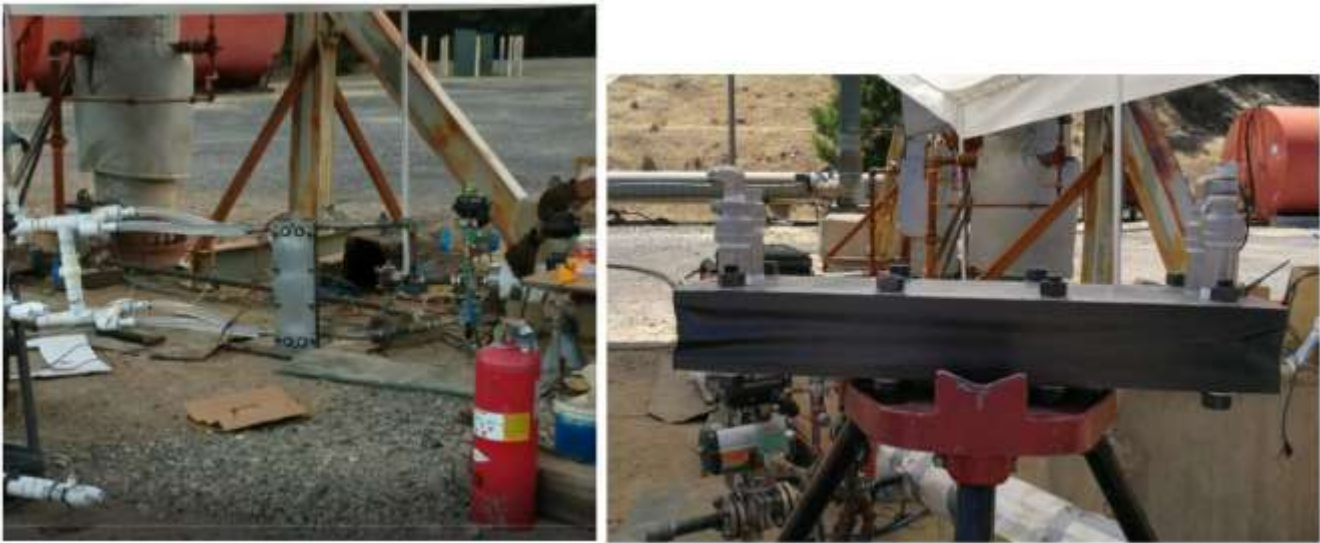
Figure 6: Bottle Rock Geothermal Field: Wellhead, Pipes, and Manifolds Adapted to Connect to the 200 W 5-Layer TEG Lab Apparatus, July 2019.
