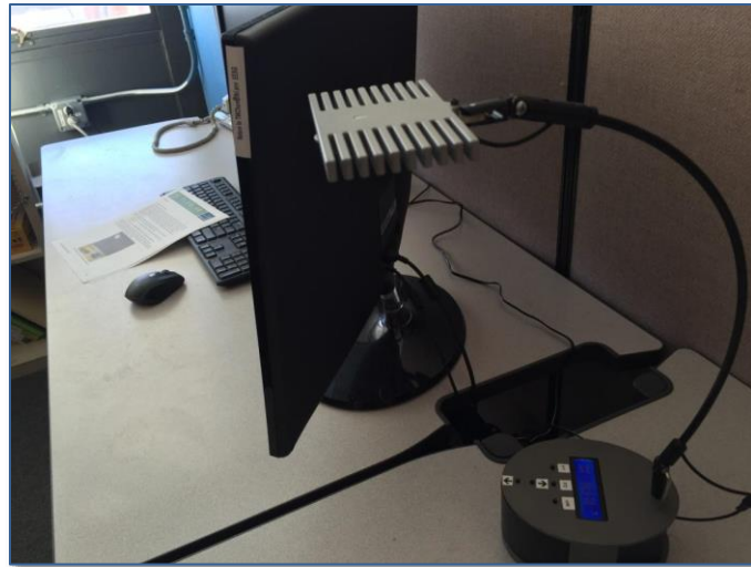
Figure 17: Initial Readings-At-Desk Controller Prototype Installed in FLEXLAB®
